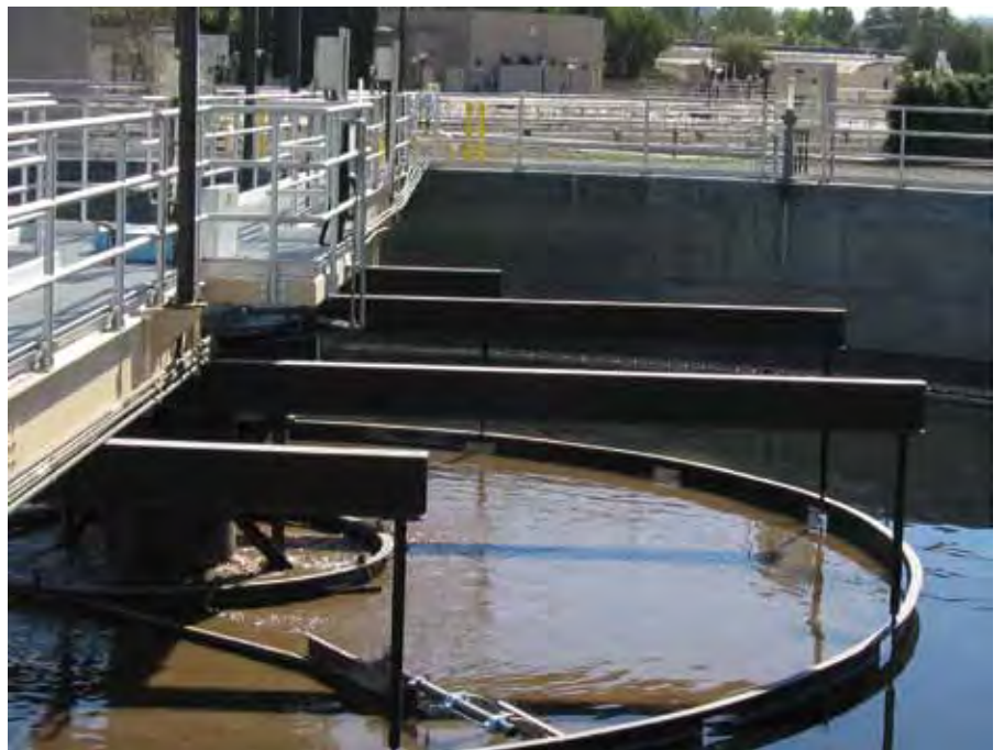
High-rate circular clarifier at the Michelson Water Recycling Plant. Current expansion of this plant, to be completed in 2012, will increase capacity from approximately 18 to 28 million gallons per day of recycled water.
