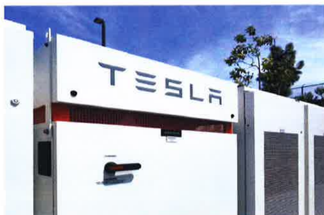
Tesla Battery Station
