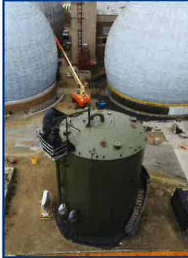
Digester Gas Holding Tank
