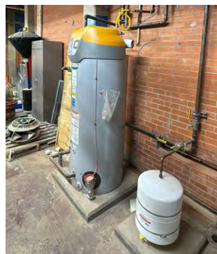
Natural gas fueled water heater and pump.
