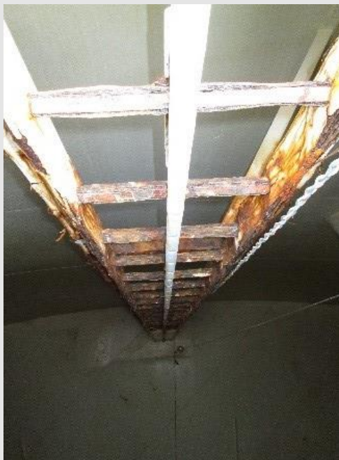
Severe corrosion on interior ladder
