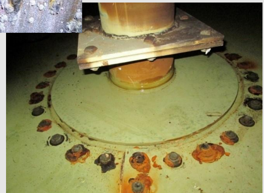
Corrosion of fasteners at the base of a bolted steel tank roof support center column
