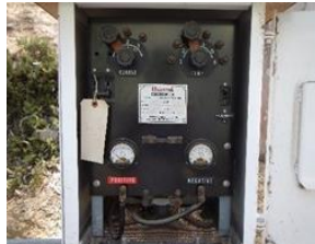
Impressed Current Rectifier
