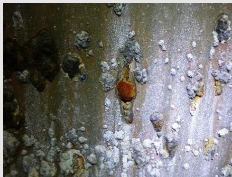
Corrosion nodules observed on the interior tank wall
