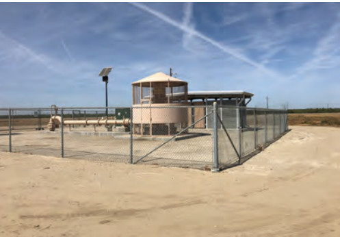
Stockdale West Well Pump
