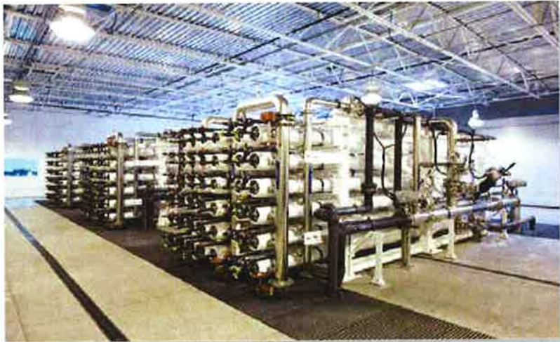
Wells 21 & 22 Water Treatment Plant
