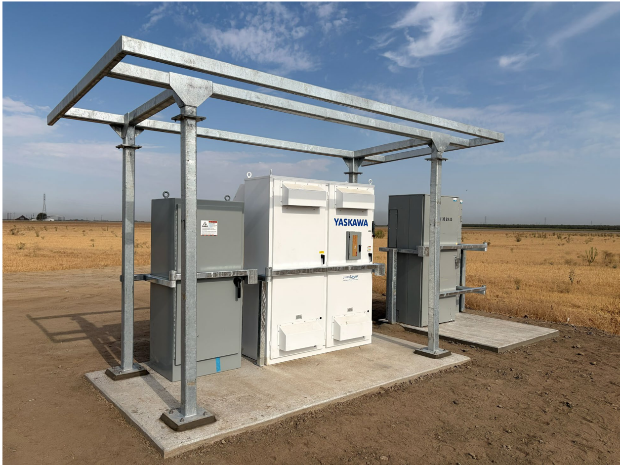
SN-2: Electrical Gear Installation with Shade Structure and Security Protection
