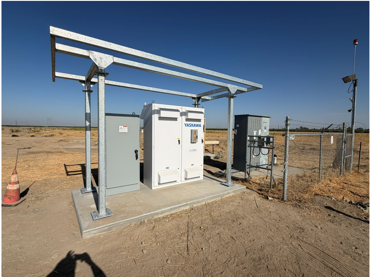
WE-AG: Electrical Gear Installation with Shade Structure
