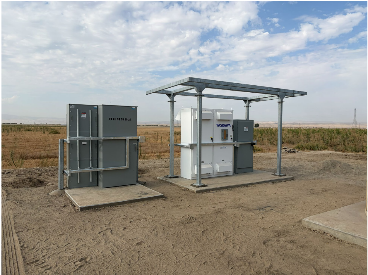
SN-1: Electrical Gear Installation with Shade Structure and Security Protection
