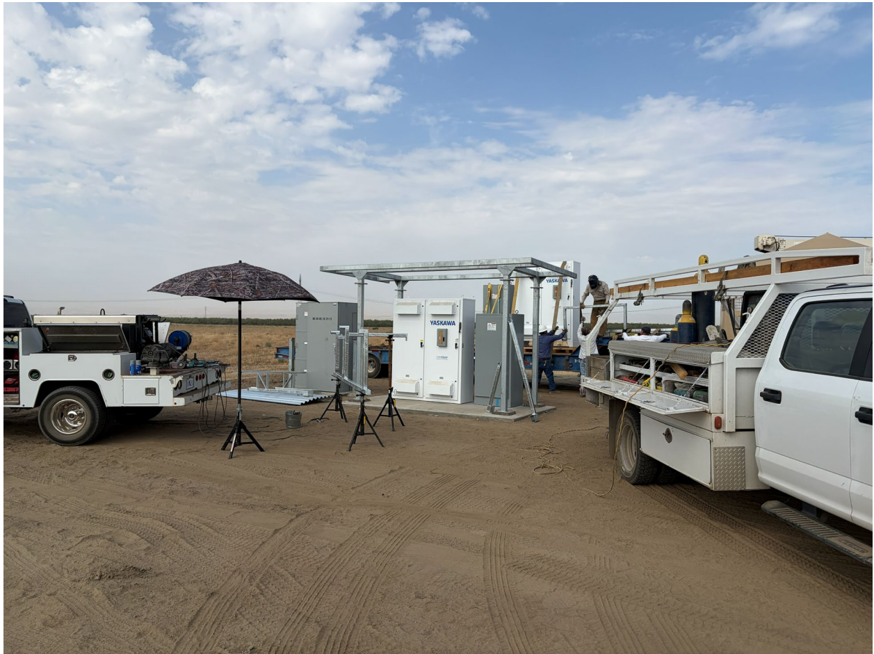
WE-1: Electrical Gear Installation with Shade Structure and Security Protection
