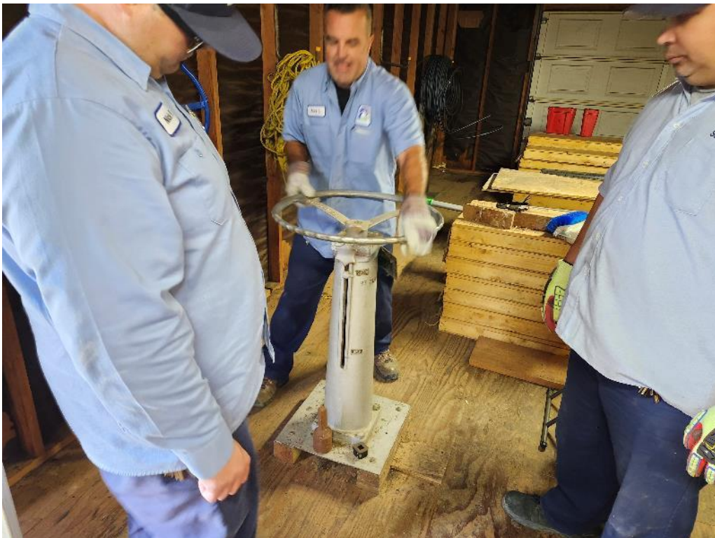
Photo 8. Cycling one of the downstream 30-inch blowoff butterfly valves.
