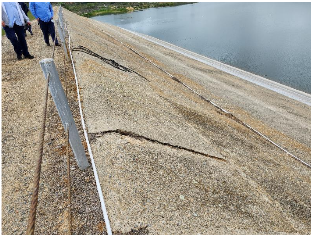
Photo 3. Crack in the upstream concrete liner.
