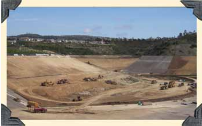
IRWD converted the San Joaquin Reservoir from drinking water storage to a one billion gallon recycled water storage facility in 2004. Here, crews regrade the reservoir to prepare for the installation of a new lining.
