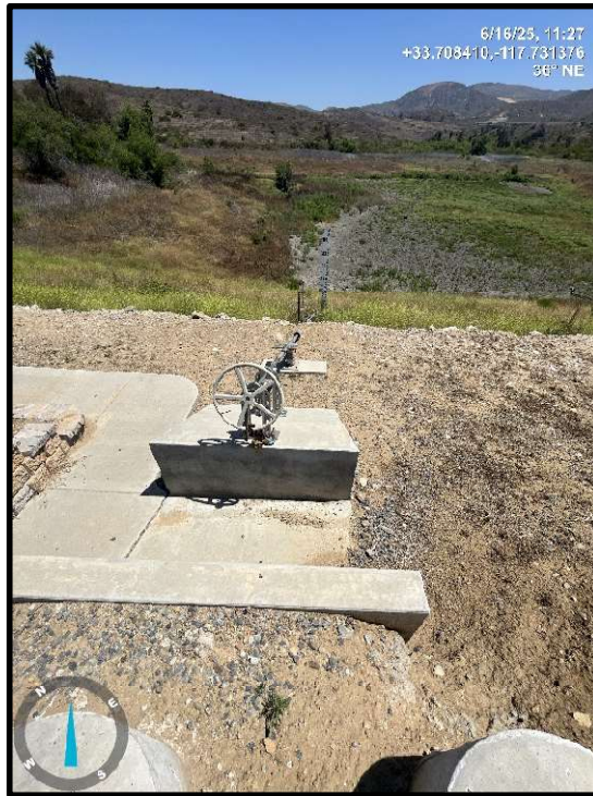
Photo 4) Syphon reservoir, outlet works, and reservoir staff gauge.
