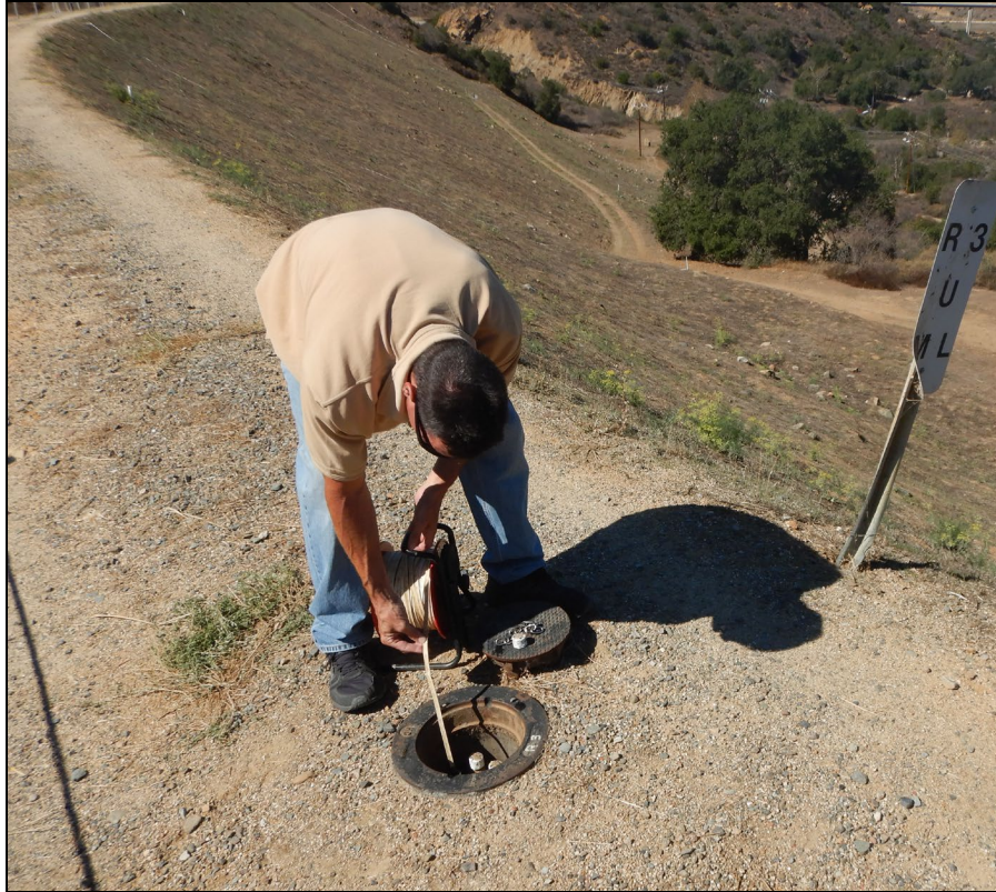
Photograph 3: View of water level meter used to take readings in Piezometer R-3 Middle at Santiago Creek Dam.
