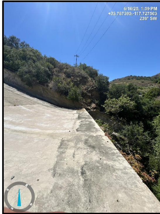
Photo 17) View of spillway flip bucket from right side of spillway channel. Note missing section of concrete wall at the left end of the spillway chute and flip bucket.
