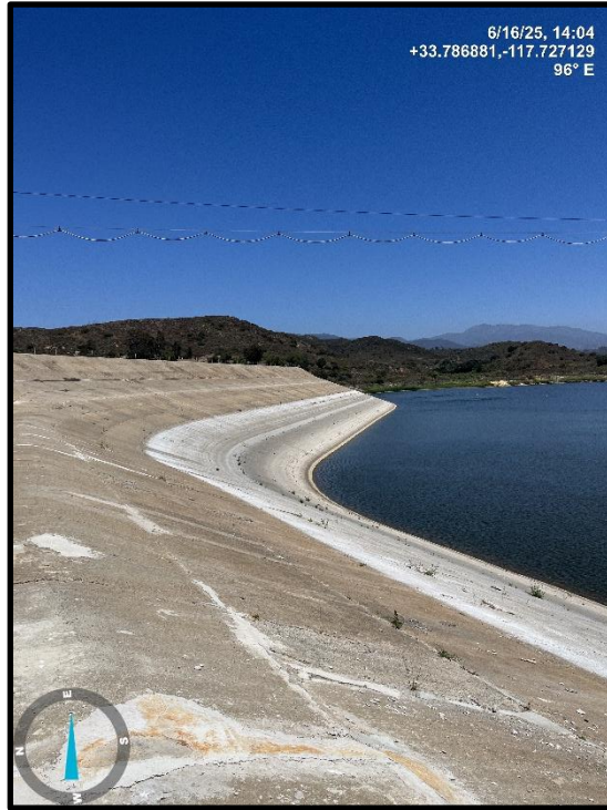
Photo 7) Upstream face looking towards right abutment. Note minor vegetation in panel joints.
