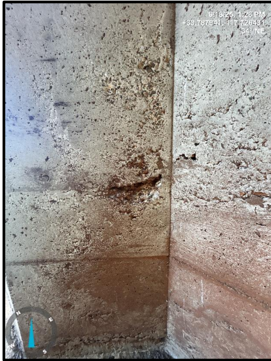
Photo 19) Concrete spalling within dissipator structure.
