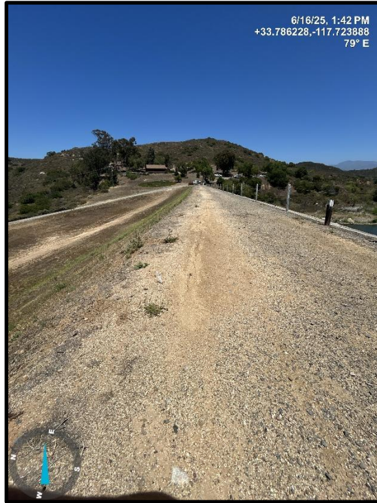
Photo 13) Crack Location 1 along dam crest.
