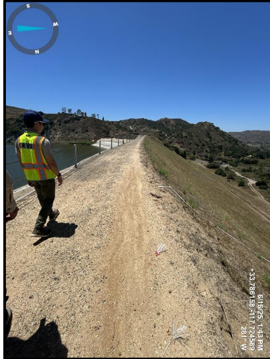
Photo 14) Crack Location 2 along dam crest.
