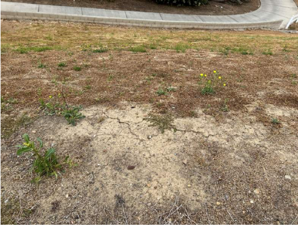
Figure 2: Sand Canyon Dam desiccation type crack near left groin along golf cart path.
