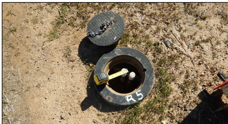
Photograph 4: View of 1-inch diameter PVC Standpipe Piezometers R-5 Lower and R-5 Upper.
