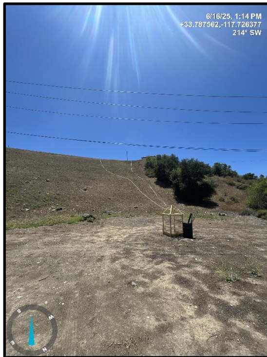
Photo 6) View of downstream face near left abutment area. Note recent vegetation removal.
