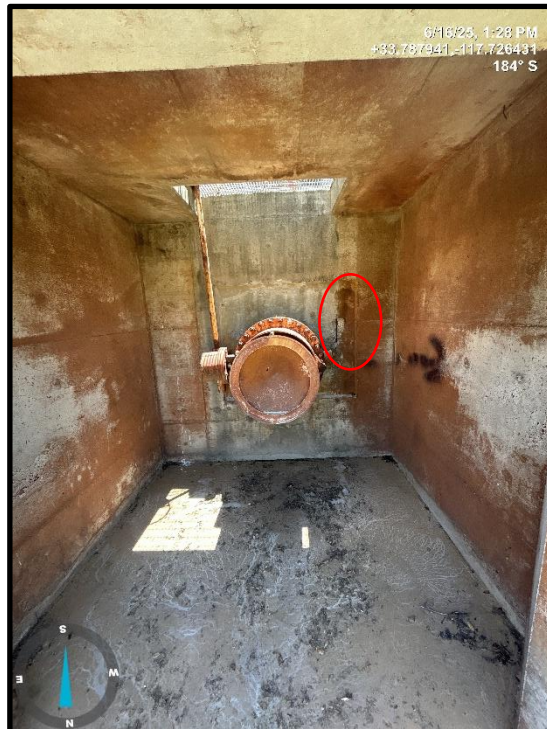
Photo 18) Emergency blowoff valve within dissipator structure. Location of exposed rebar shown in red circle.
