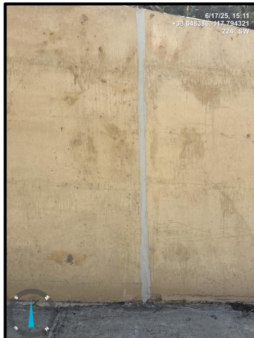
Photo 24) Vertical wall joint open 1/2" max between wall panels L2 and L3. Note recent repair of joint.
