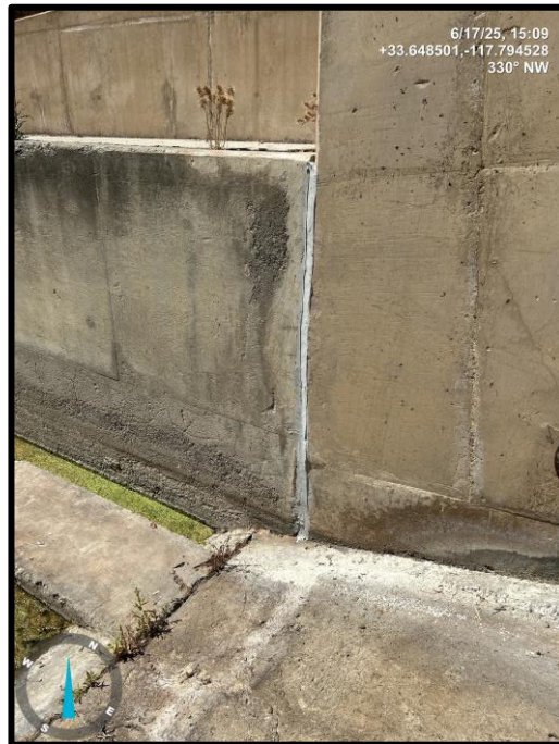
Photo 35) Previously repaired spillway vertical wall joint.
