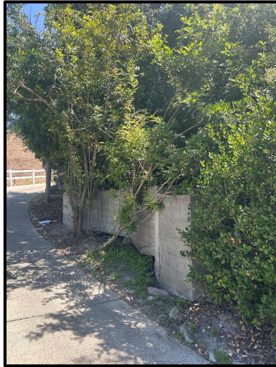
Photo 3) Abandoned irrigation weir box. Note seepage surrounding the box.
