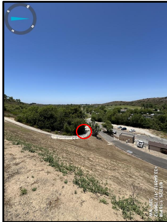
Photo 5) Downstream face of dam near left abutment. Note abandoned irrigation weir box.
