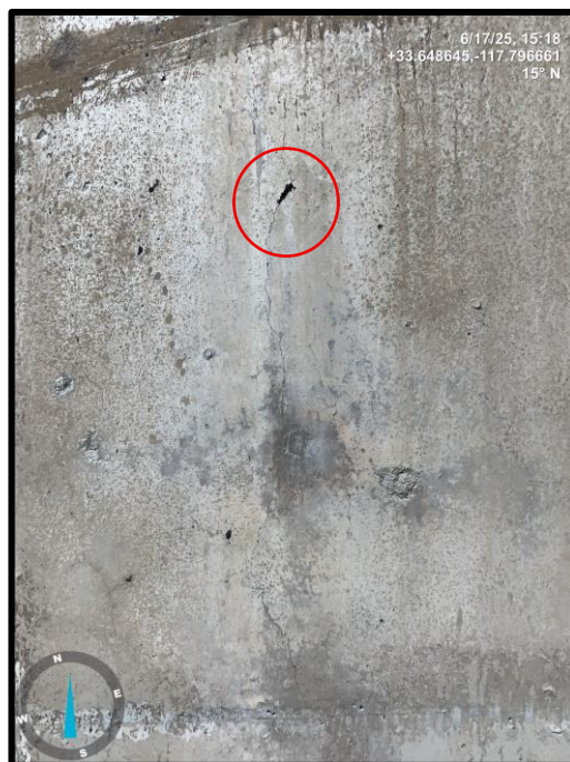
Photo 16) 1/8" crack and 2" x 3/4" concrete popout wall panel R1.
