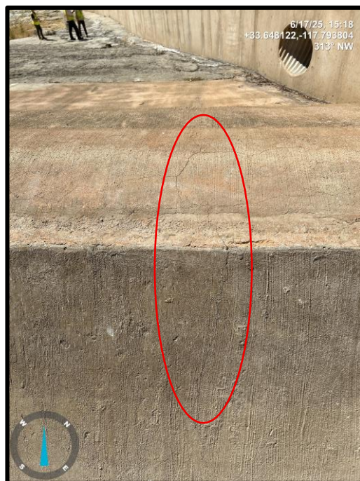
Photo 12) Minor cracking along upstream face of weir.
