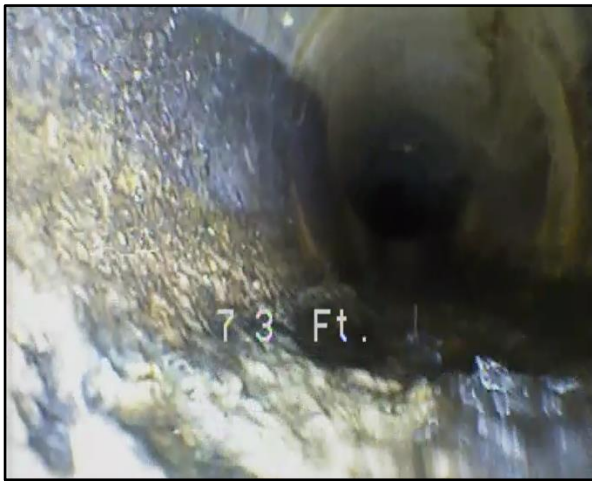
Photo 1 – STA 00+07: Pipe is in good condition with 75% staining on its walls (typical).
