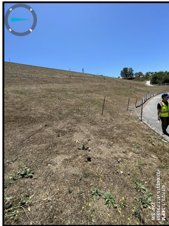
Photo 8) Minor rodent activity on the downstream toe near the right abutment.
