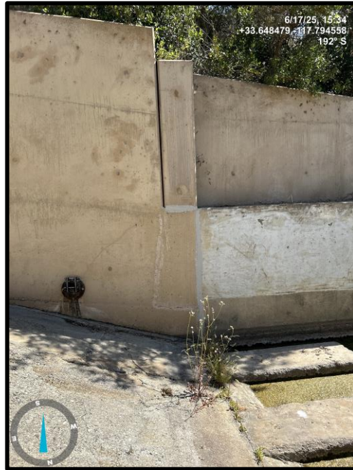
Photo 37) Previously repaired spillway vertical wall joint. Note spillway drain and vegetation..
