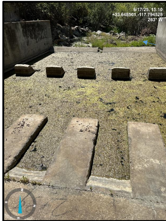
Photo 11) Close up view of spillway stilling basin. Note brush/tule growth downstream and two spalling baffle blocks on the right.
