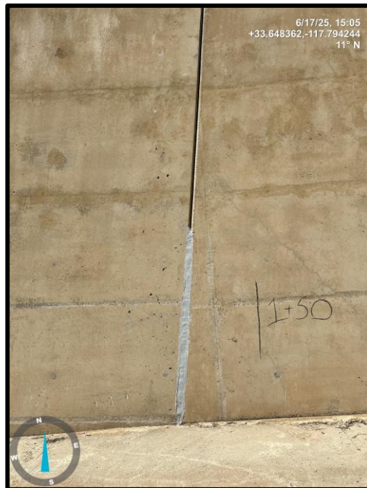
Photo 26) Vertical wall joint open ½" max between wall panels R2 and R3. Note previous repair of bottom half of joint.
