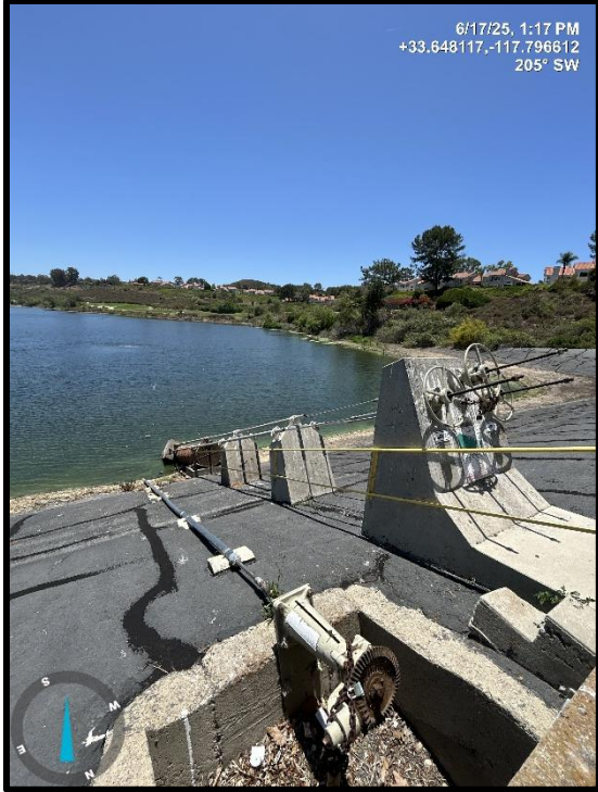
Photo 14) View of the gate valve system.
