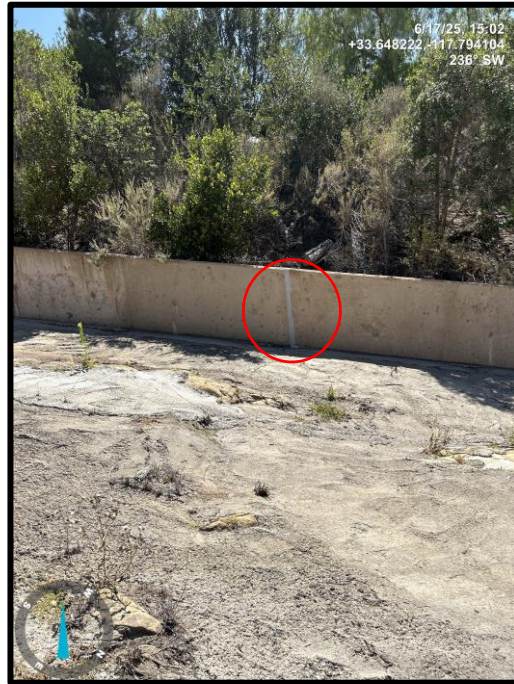
Photo 19) View of spillway wall panels L1 and L2. Note previously repair of joint.
