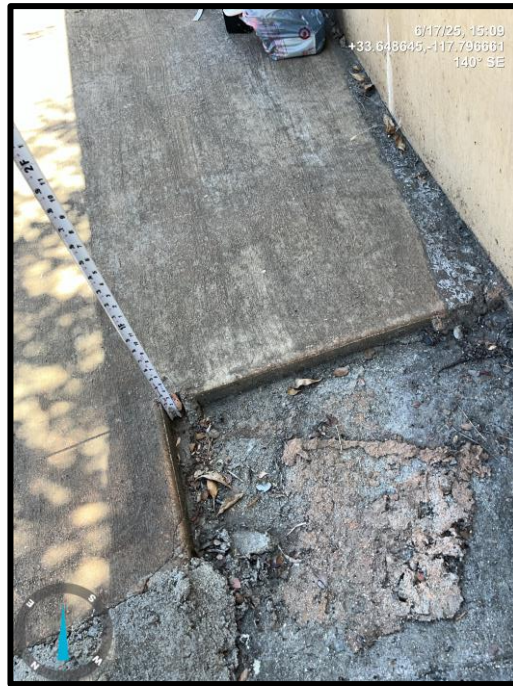
Photo 1) ½” slab joint offset near toe of spillway ogee weir.
