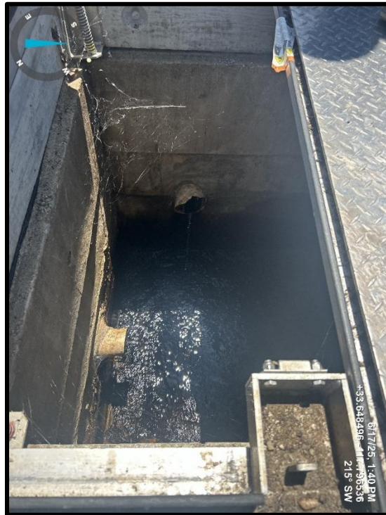
Photo 17) Seepage at left subdrain. Right subdrain was dry.
