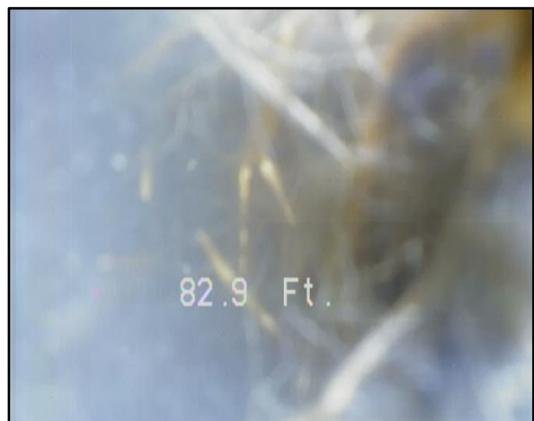
Photo 4 – STA 00+82: Root ball inside pipe.
