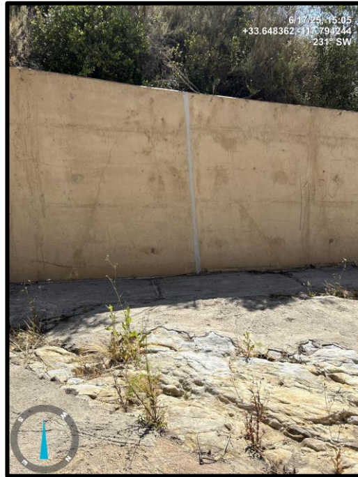
Photo 23) View of spillway wall panels L2 and L3. Note recent repair of joint.
