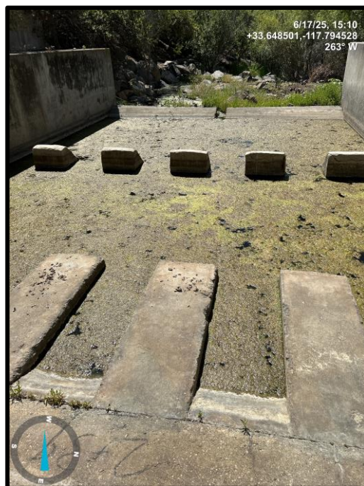
Photo 36) Spillway stilling basin. Note 1/2" cracks on right two concrete baffles.
