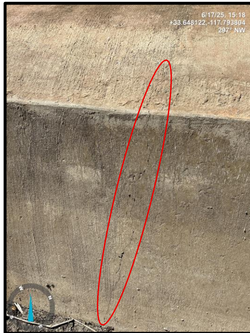
Photo 13) Minor cracking along upstream face of weir.
