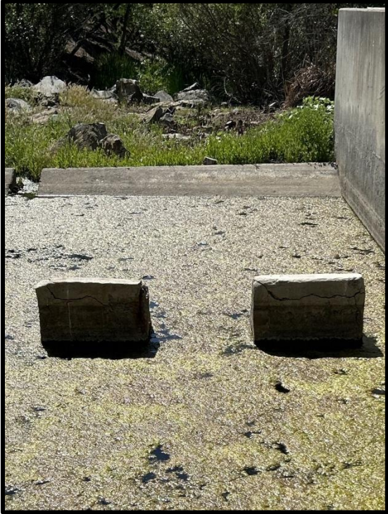
Photo 13) View of the gate valve system.
