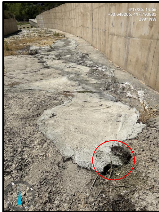
Photo 5) 5” depth void at previous spillway repair.
