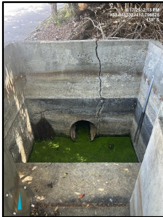
Photo 4) Abandoned irrigation weir box. Note pooled water.
