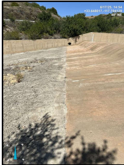
Photo 2) View of spillway ogee weir and unlined spillway channel transition looking northeast.
