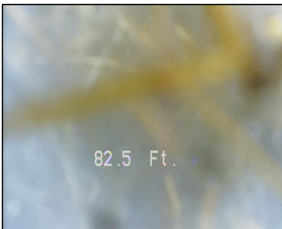
Photo 3 – STA 00+82: Root ball inside pipe.
