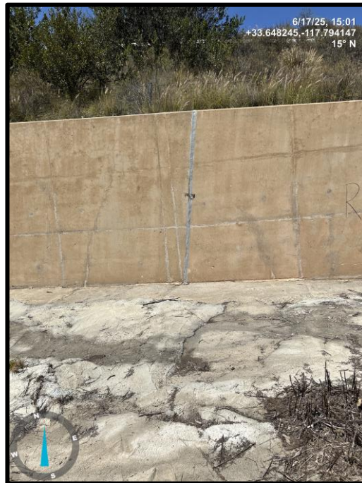
Photo 15) Previously repaired joint.
