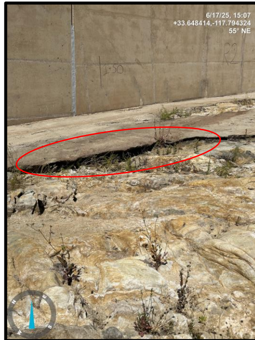
Photo 29) 12" max height x 12" max depth spillway floor undermining.
