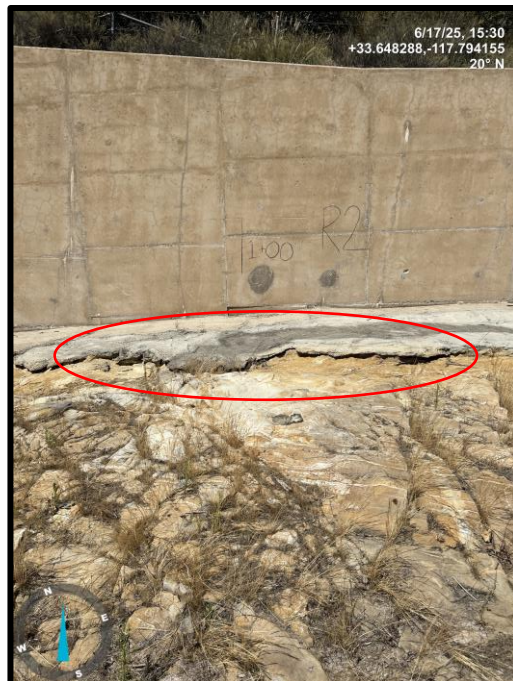
Photo 18) 6" Height x 8" Depth spillway floor undermining.
