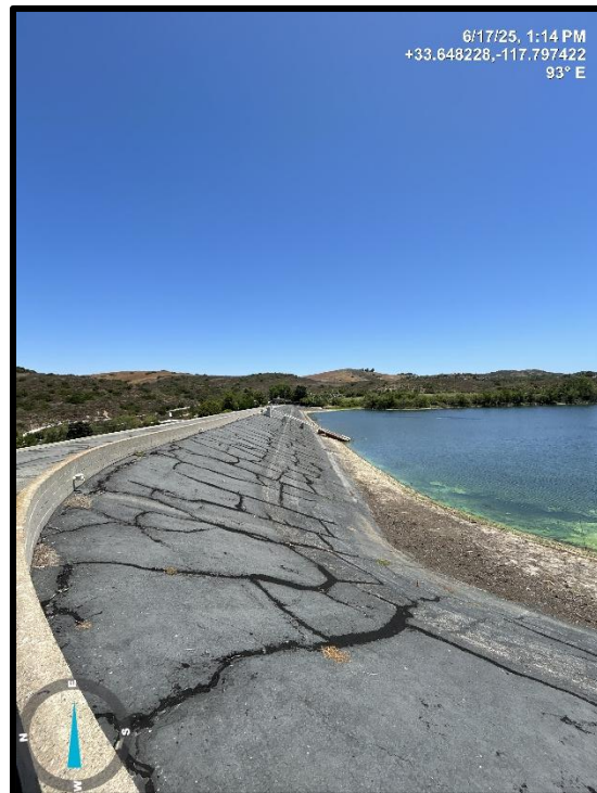
Photo 2) AC-lined upstream face looking towards right abutment. Note cracks along face.
