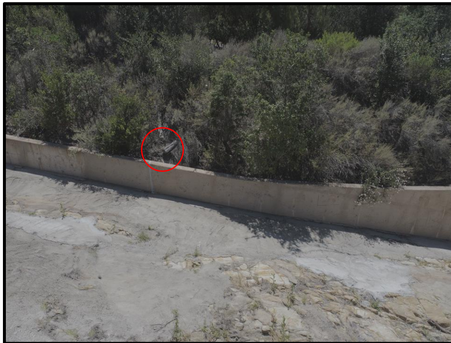
Photo 20) View of spillway wall panels L1 and L2. Note previous repair of joint.
