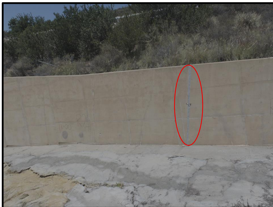
Photo 14) View of spillway wall panel R1 and R2. Note previous repair of joint.
