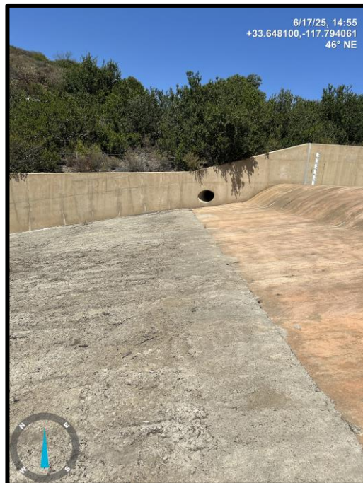
Photo 4) View of spillway ogee weir and unlined spillway channel transition looking northeast. Note 2' diameter corrugated metal pipe.
