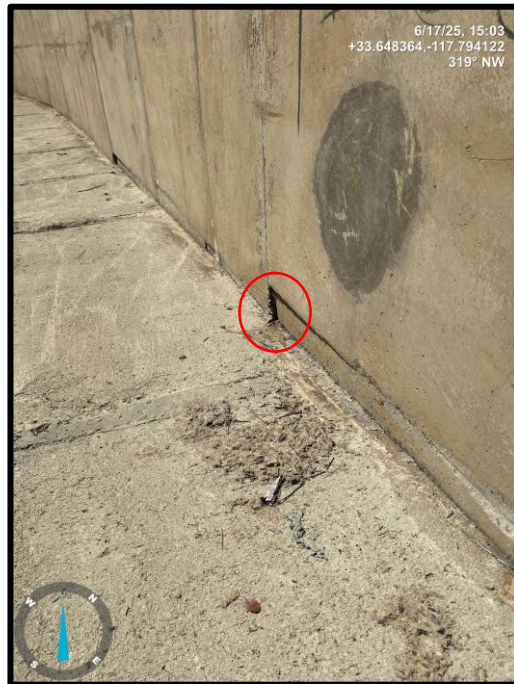
Photo 21) 1” offset at bottom of spillway wall panel R2.
