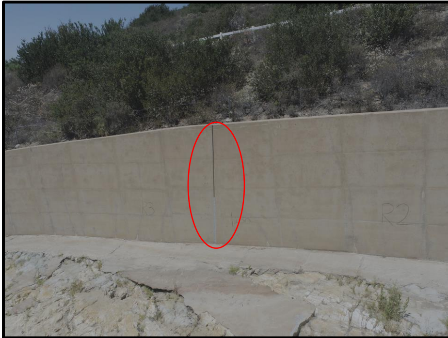
Photo 25) View of spillway wall panels R2 and R3. Note previous repair of bottom half of joint.
