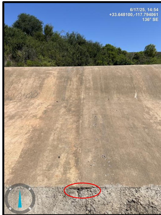
Photo 3) 1" slab joint offset at spillway ogee weir and unlined spillway channel transition.
