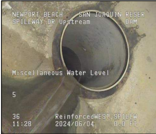
Photo 32 – STA 00+00: Water flowing out of the pipe.
