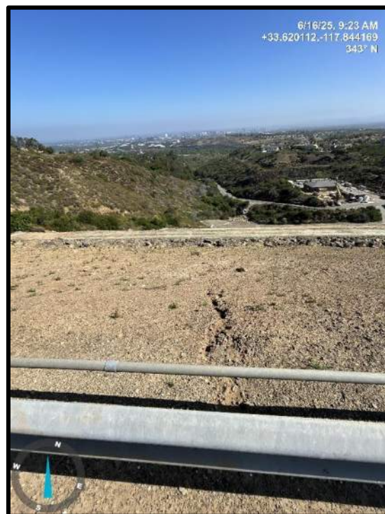
Photo 10) Minor rill erosion on the downstream face.
