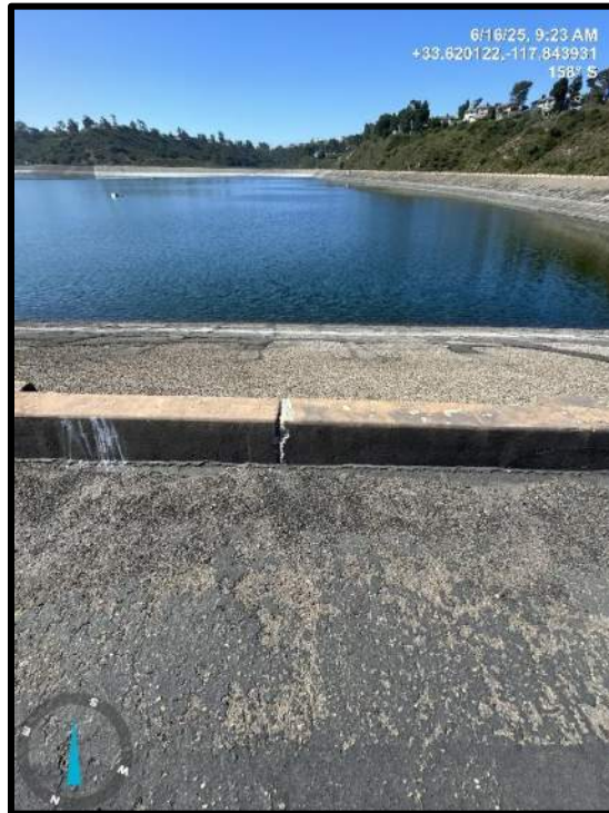
Photo 5) Minor cracks and spalling at concrete curb joints.
