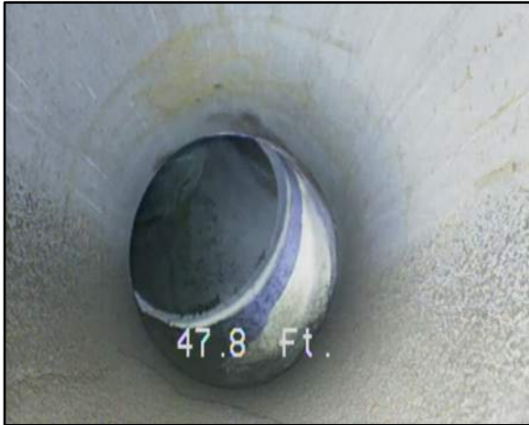
Photo 3 – STA 00+47: Bend in the pipe.
