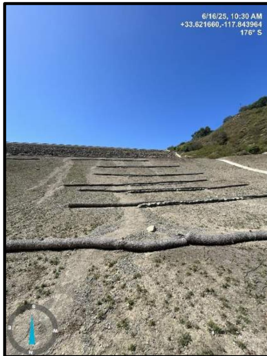
Photo 14) Looking at downstream slope from the toe of dam. Note minor rill erosion.
