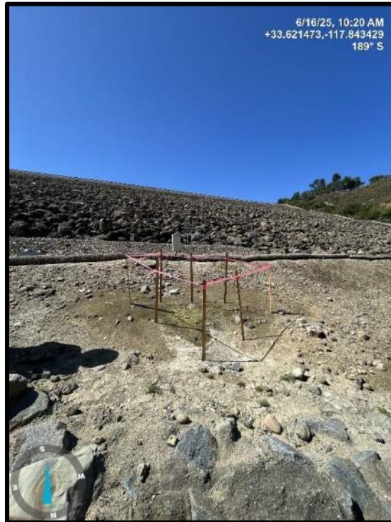
Photo 19) Wet spot observed on downstream face of dam.
