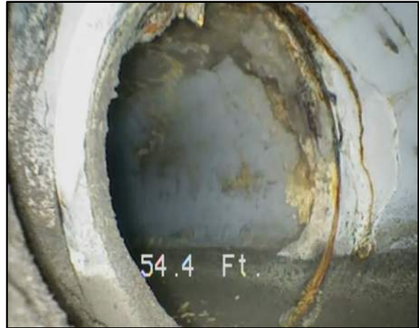
Photo 4 – STA 00+54: Staining of the joint.
