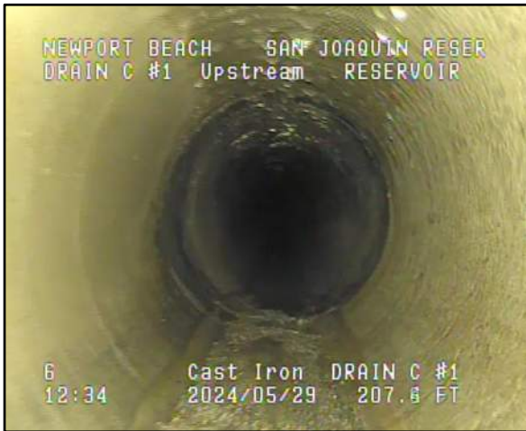
Photo 17 – STA 02+07: Debris on the bottom of the pipe.
