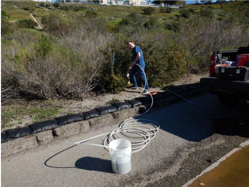
Photograph 2: View of flushing process being performed in Piezometer CP-3B at San Joaquin Dam.
