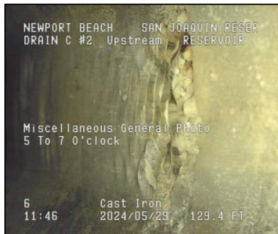
Photo 22 – STA 01+29: Lining damaged from 5 to 7 o'clock.
