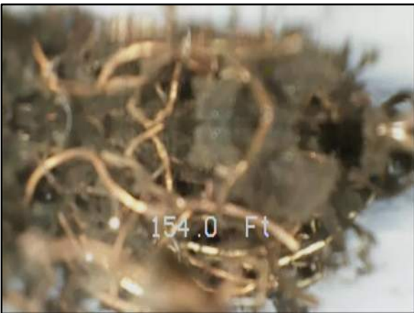
Photo 30 – STA 01+54: Root ball in the pipe.
