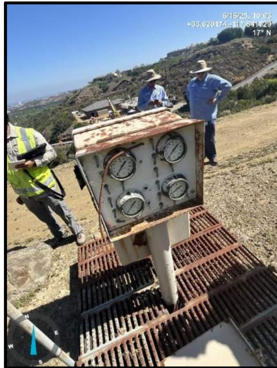
Photo 17) Relief valve gauge behind pneumatic piezometer terminal box. Note significant corrosion.
