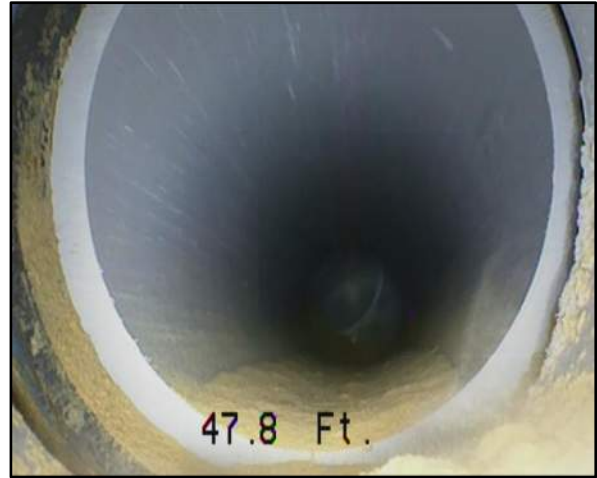
Photo 12 – STA 00+04: Sand debris on the bottom of the pipe.
