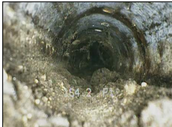
Photo 31 – STA 01+64: Debris in the pipe and the end of the survey.
