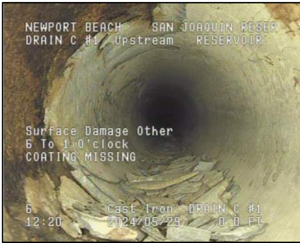
Photo 15 – STA 00+00: Failed liner.
