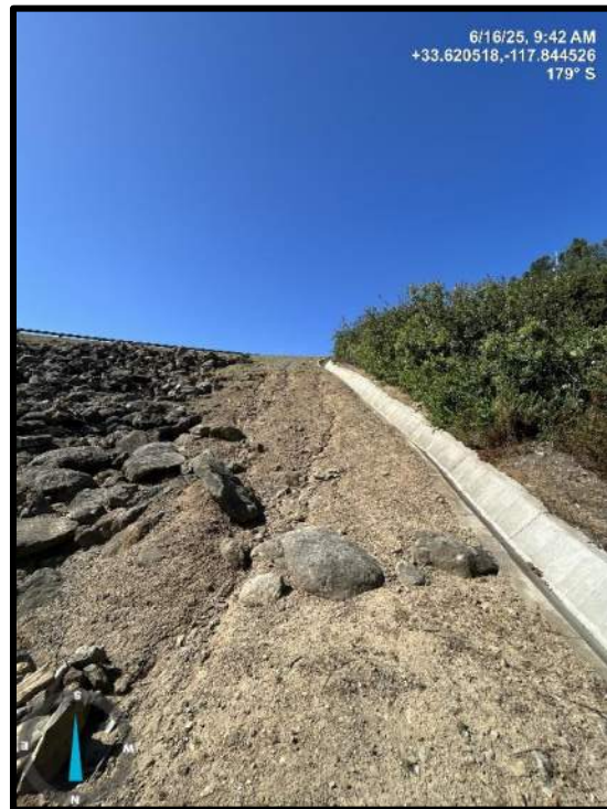
Photo 9) Minor rill erosion along the left groin between the top downstream bench and the dam crest.
