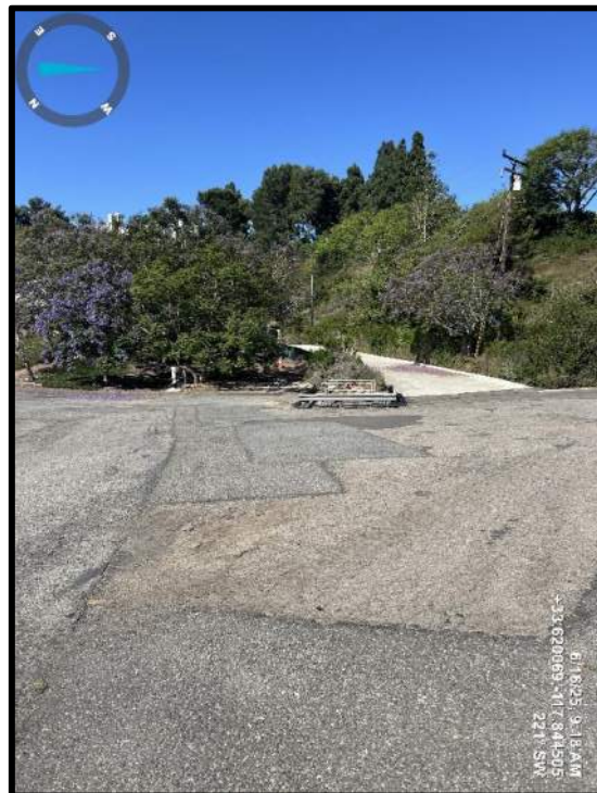
Photo 4) Recent repair of AC pavement cracking on crest looking towards the left abutment.
