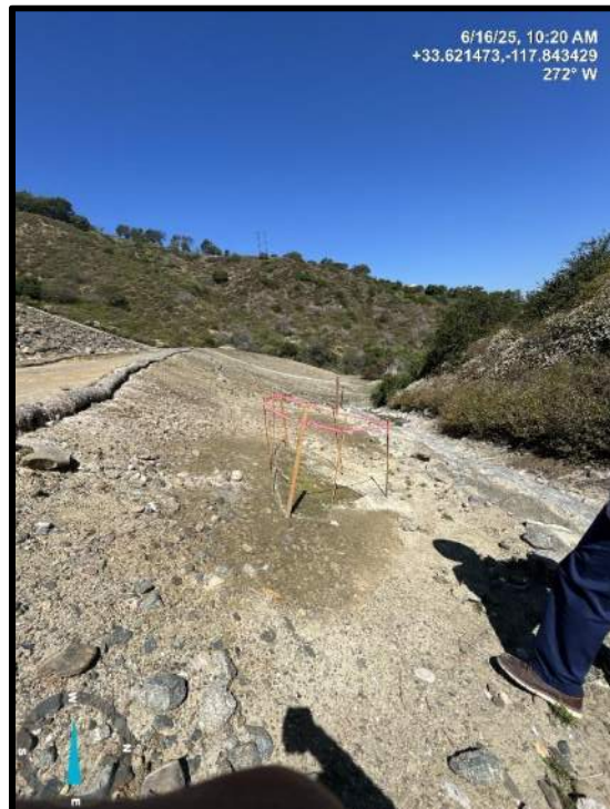
Photo 28) Newly identified wet spot with stakes marking original bounds.
