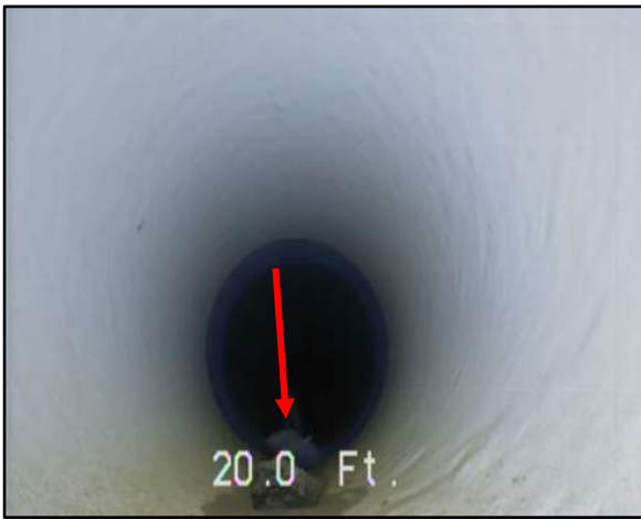
Photo 9 – STA 00+20: Rock on the bottom of the pipe.
