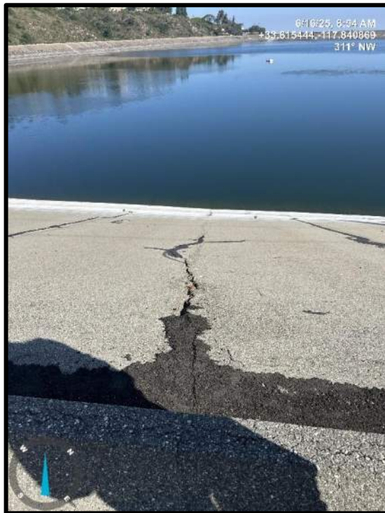
Photo 22) Cracks in the upstream portion of the reservoir liner filled with cold patch asphalt.
