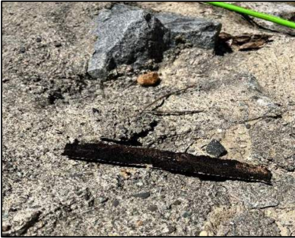
Photo 28 – Mineral encrustation layer on the bottom of the pipe.
