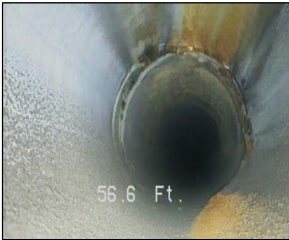
Photo 5 – STA 00+56: Staining on the pipe ceiling.
