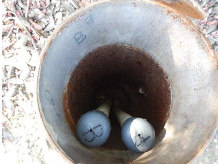
Photograph 5: View of 1-inch diameter PVC Standpipe Piezometers CP-2A & CP-2B at San Joaquin Dam.
