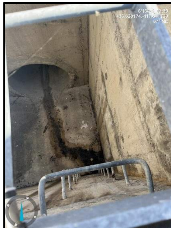
Photo 24) Minor seepage at the right spillway drop inlet.
