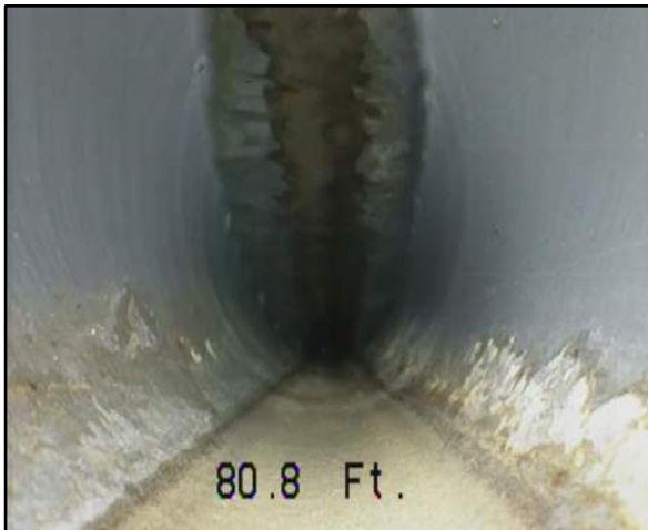
Photo 13 – STA 00+80: Air bubble and staining on the walls of the pipe.
