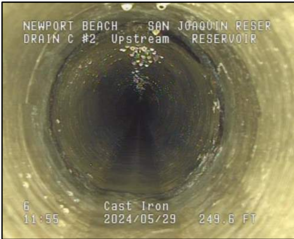
Photo 25 – STA 02+49: Corrosion at pipe joint.
