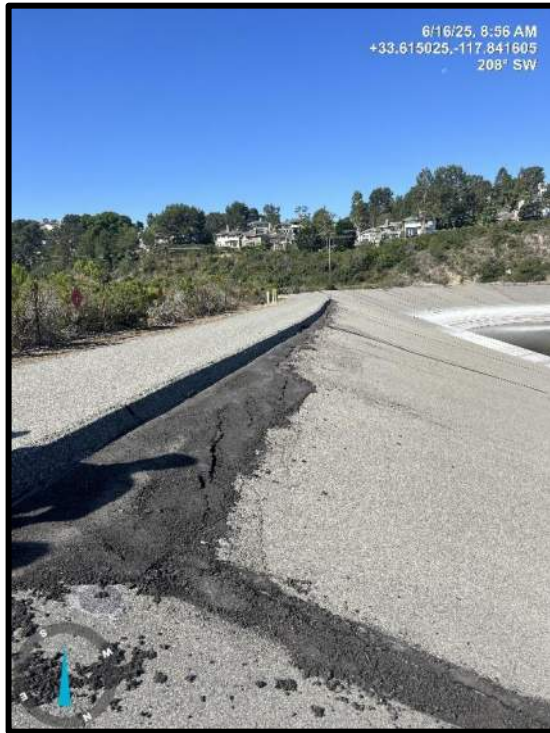
Photo 21) Cracks in the upstream portion of the reservoir liner filled with cold patch asphalt.
