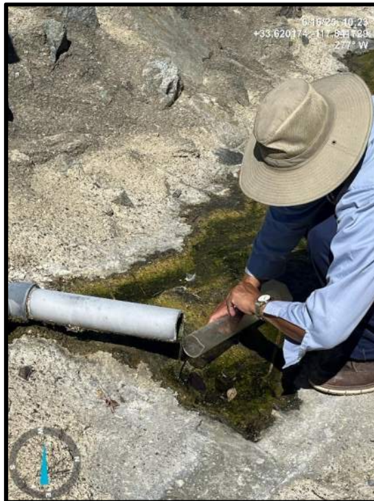
Photo 26) Taking seepage reading at Right Groin Drain.
