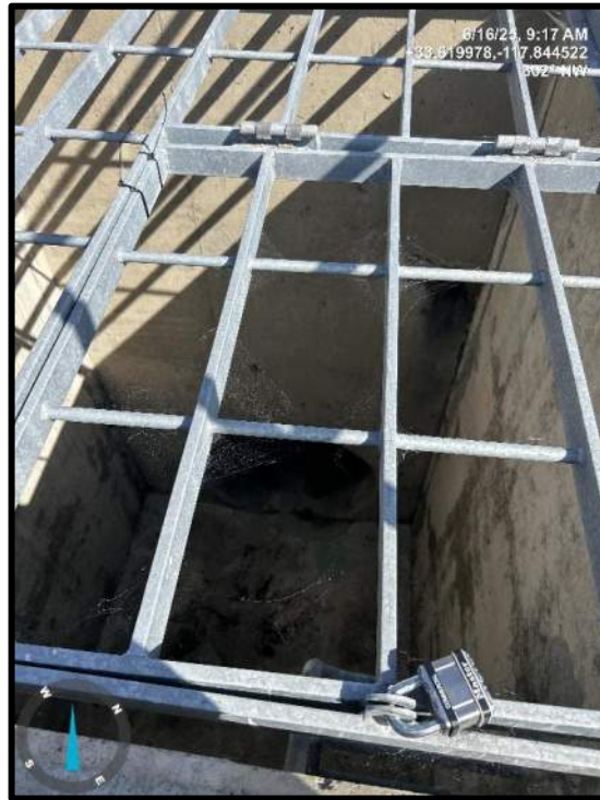
Photo 23) Bottom of right spillway drop inlet. Note water stain.
