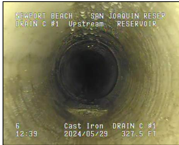
Photo 18 – STA 03+27: Debris on the bottom of the pipe.
