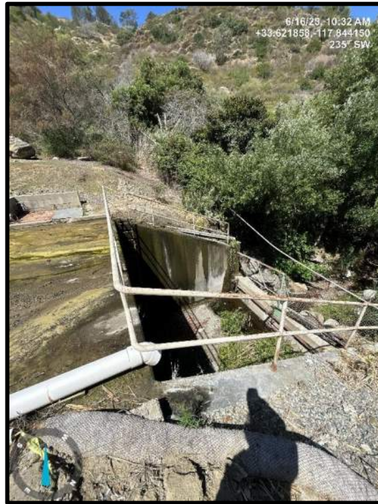
Photo 15) Energy dissipator structure. Note significant corrosion on handrails and ladder. Note the D/S Toe and Floor Drain outflow pipe.
