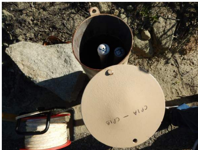
Photograph 4: View of 1-inch diameter PVC Standpipe Piezometers CP-1A & CP-1B at San Joaquin Dam.
