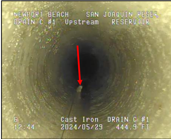
Photo 19 – STA 04+44: Rock at bottom of the pipe.
