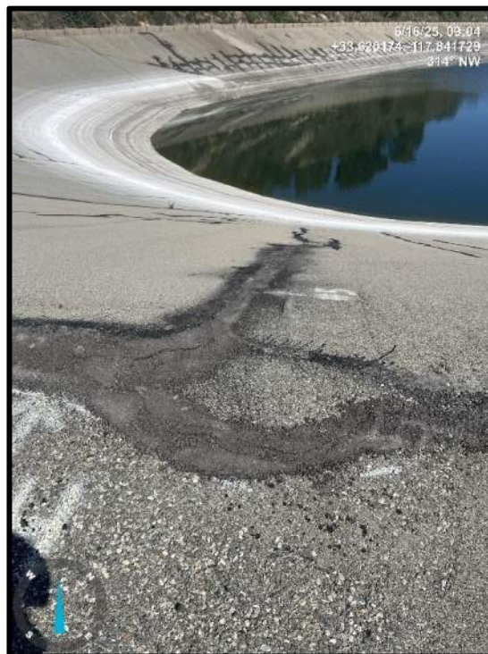
Photo 20) Cracks in the upstream portion of the reservoir liner filled with cold patch asphalt.
