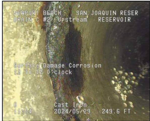
Photo 26 – STA 02+49: Closeup of corrosion at pipe joint.
