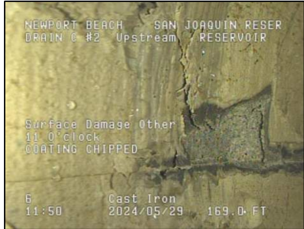
Photo 24 – STA 01+69: Cracks in lining at 11 o'clock.
