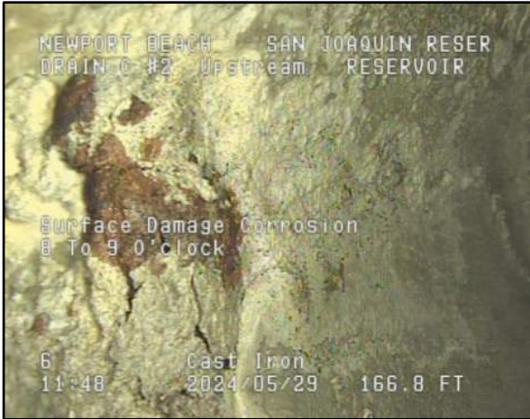
Photo 23 – STA 01+66: Lining failure and possible corrosion from 6 to 9 o'clock.
