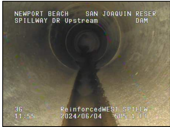
Photo 35 – STA 05+05: End of the survey due to the steepness and slipperiness of the pipe.
