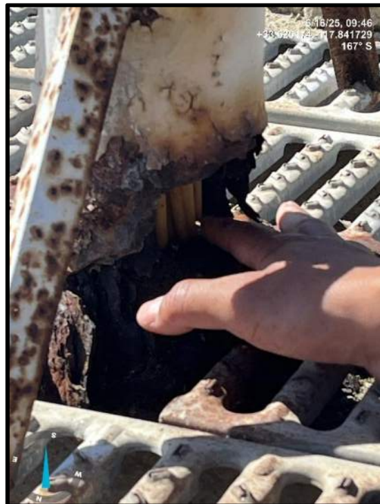
Photo 18) Exposed pneumatic piezometer tubing. Note significant corrosion and severed tube.
