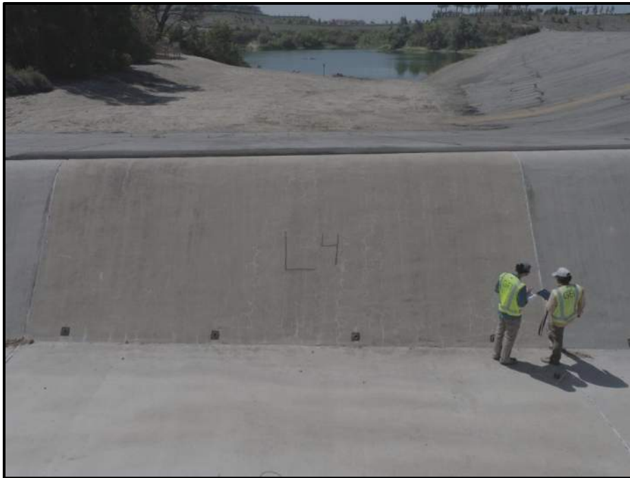
Photo 6) Minor alligator cracking and efflorescence staining throughout panel L4.
