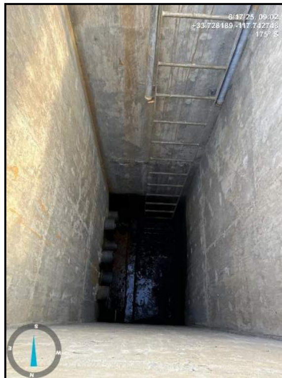
Photo 18) Seepage drain-pipe outfalls at the bottom of the seepage vault downstream of dam.
