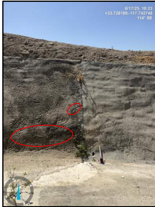
Photo 31) Vertical wall joint open \frac{1}{4} " max with 1" joint offset between wall panels L16 US and L16 DS. Note \frac{1}{2} " transverse crack and vegetation.
