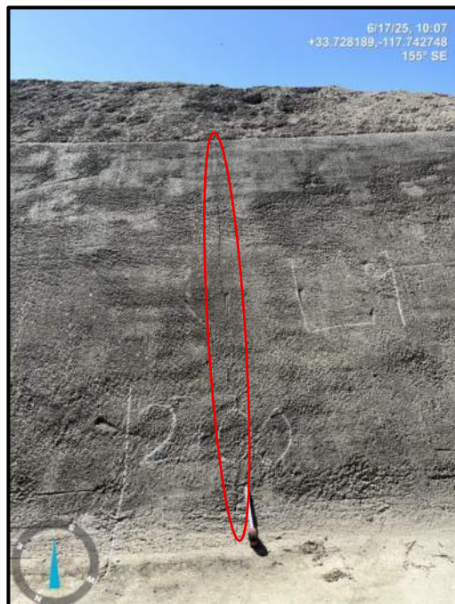
Photo 14) ¼” crack from top to bottom of wall panel L9.
