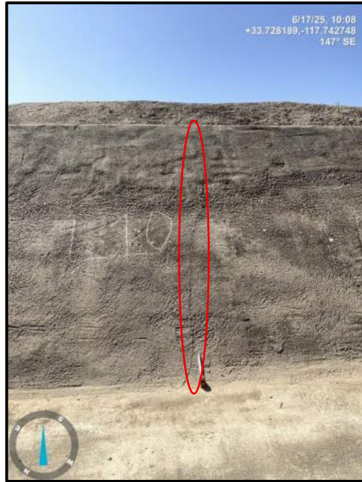
Photo 15) ¼” crack from top to bottom of wall panel L10.
