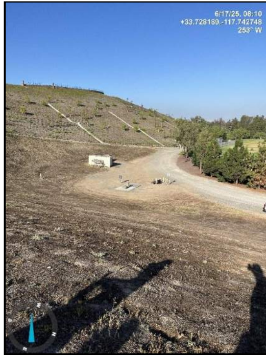
Photo 7) View along the left downstream face with view of the emergency blowoff valve.
