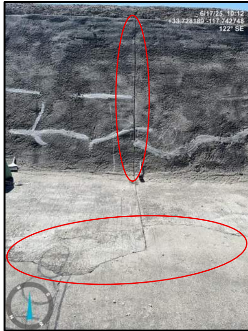
Photo 21) ¼” max slab joint opening and vertical wall joint opening at wall panels L12 and L13. Note utility trench construction joints.
