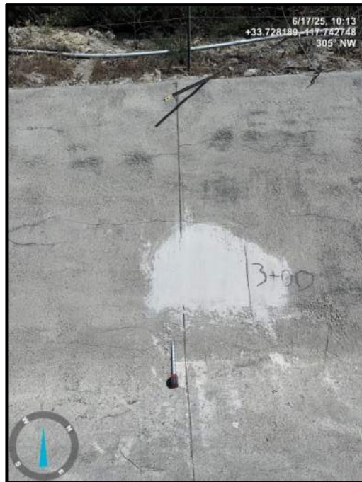
Photo 20) Vertical wall joint open 1/4" max between wall panels R12 and R13. Note previous concrete repair.
