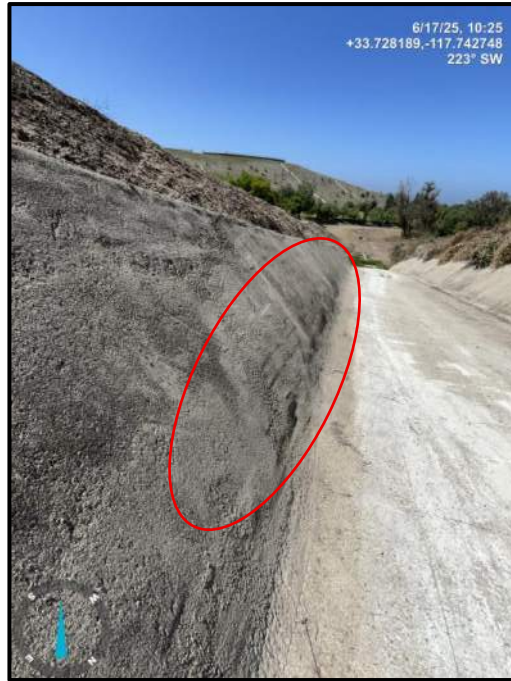
Photo 35) Bulge along wall panels L19, L20, and L21.
