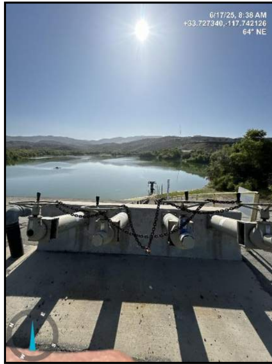
Photo 17) Upstream outlet valves.
