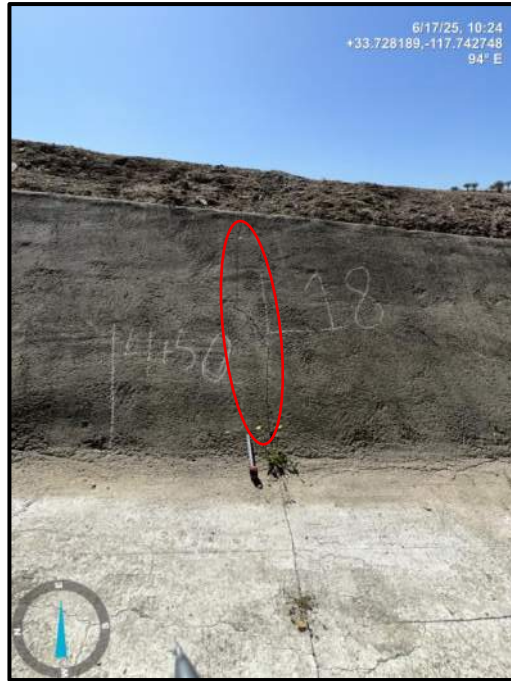
Photo 33) ½” transverse crack from top to bottom of wall panel L18.
