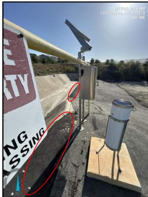
Photo 12) Previous repairs of spillway wall and dam crest separation (Typ).
