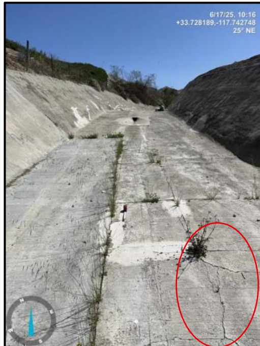
Photo 26) Existing trench from previous spillway channel repairs looking upstream. Note cracks and vegetation along construction joints.
