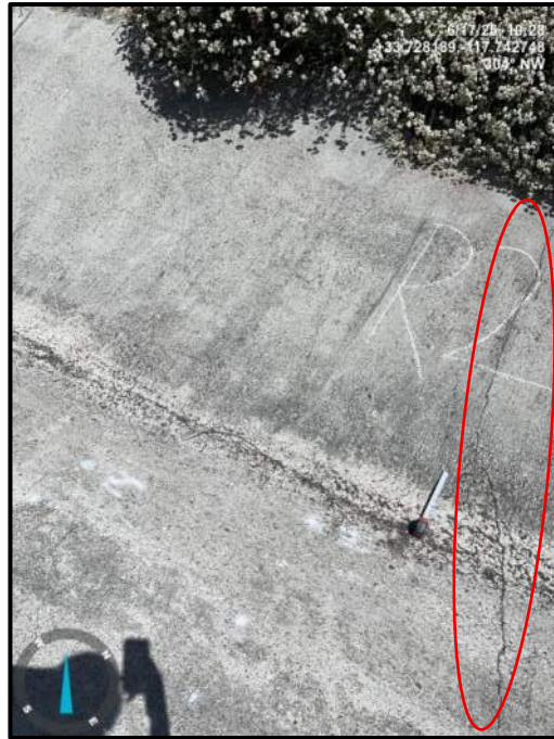
Photo 37) ¼” longitudinal crack on wall panel R20.
