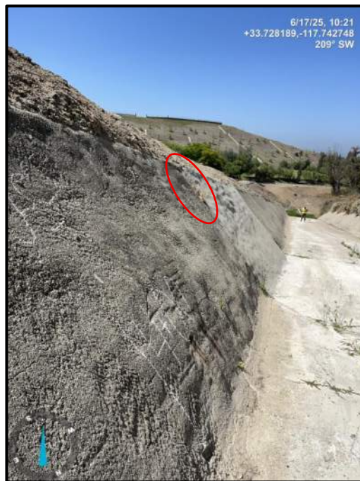
Photo 30) Vertical wall joint open ¼” max with 1” joint offset between wall panels L16 US and L16 DS. Note alligator cracking throughout panel.
