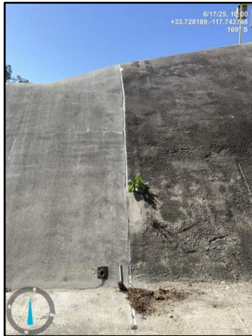
Photo 8) Vertical wall joint open ½” top to middle between wall panels L5 and L6. Note previous concrete repair and plant growth.
