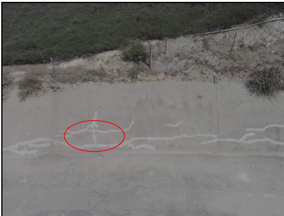
Photo 18) Existing bulge along wall panel R11. Note previous concrete repairs throughout bottom 1/3 of panel.
