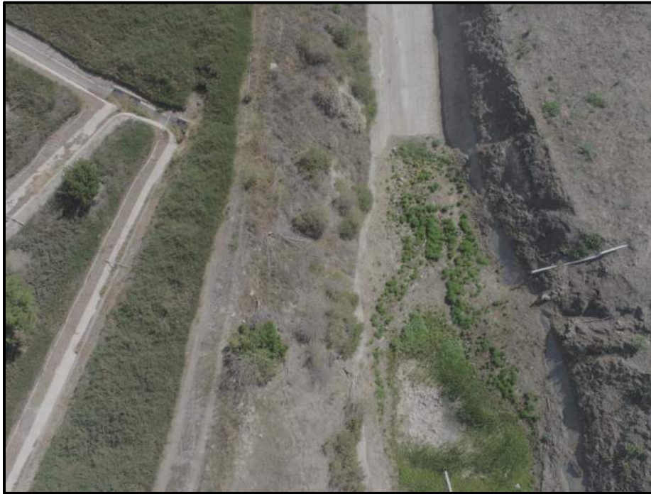
Photo 49) View of spillway stilling basin looking upstream. Note vegetation and sediment.
