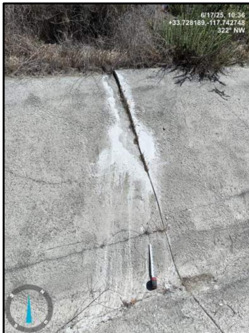
Photo 42) Vertical wall joint open \frac{1}{2} " max with 1 \frac{3}{4} " joint offset between wall panels R25 and R26. Note vegetation growth.
