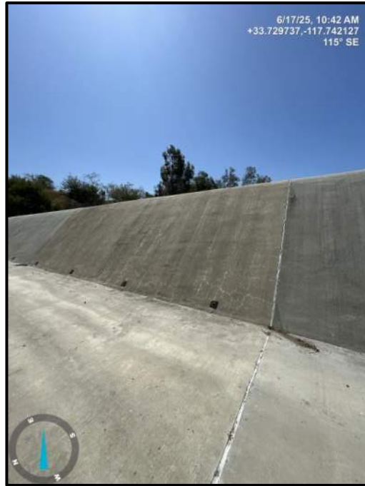
Photo 7) Vertical wall joint open ½” max between wall panels L4 and L5.
