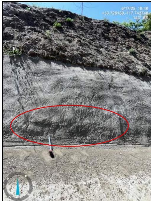
Photo 46) Concrete spall and ¼” transverse crack on wall panel L27.
