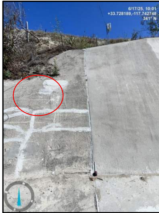
Photo 9) Vertical wall joint open 1/2" top to middle between wall panels R5 and R6. Note previous concrete repairs and 1/4" cracks.
