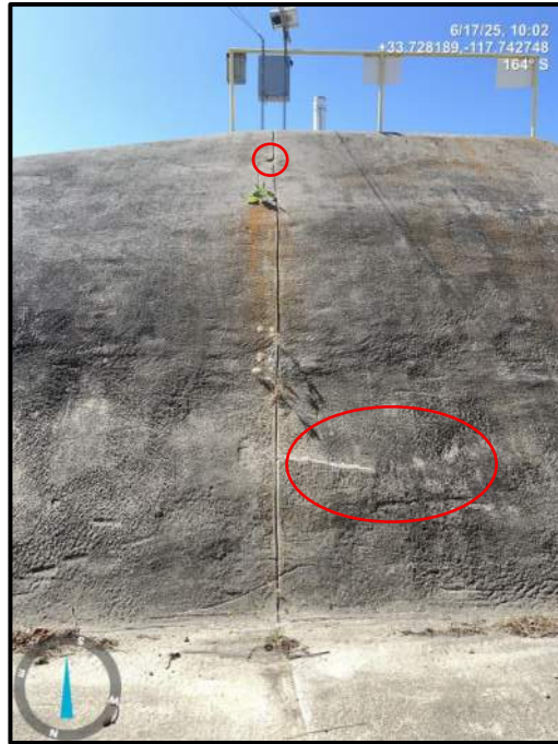
Photo 11) Vertical wall joint open \frac{1}{4} " max between wall panels L6 and L7. Note previous concrete repair and \frac{1}{4} " cracks. Concrete spall at top of joint with plant.
