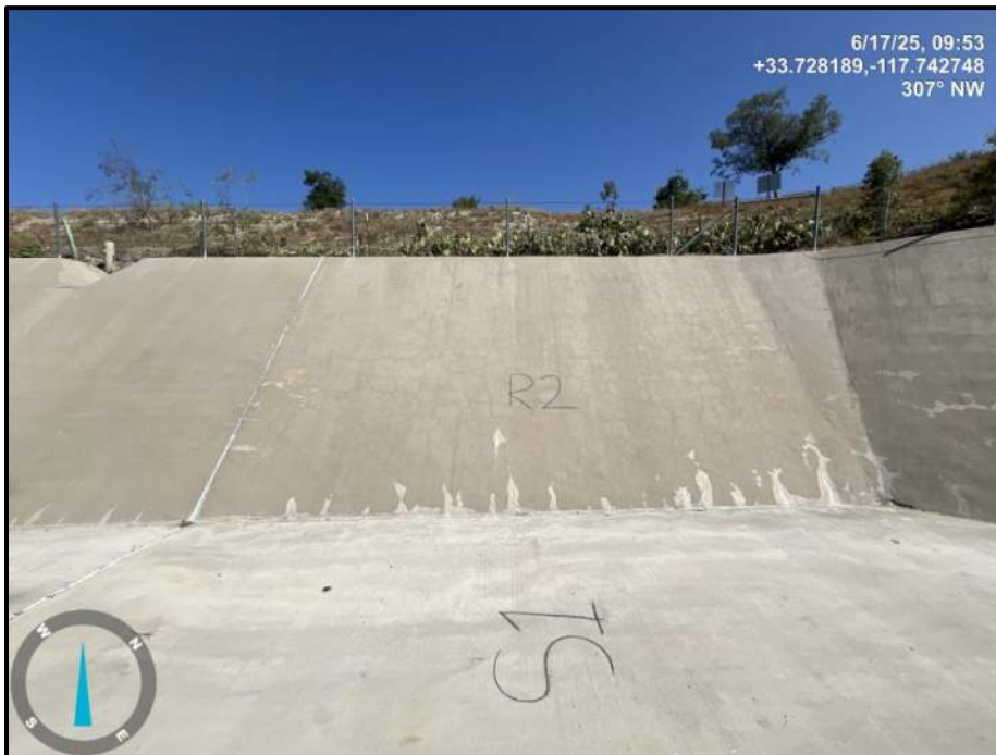
Photo 4) Alligator cracking throughout panel R2. Note efflorescence staining.
