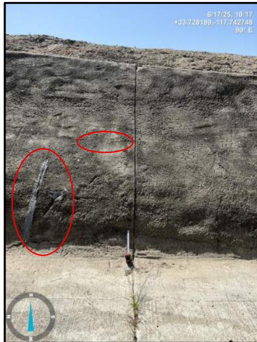
Photo 24) Vertical wall joint open \frac{1}{2} " max between wall panels L14 and L15. Note \frac{1}{2} " transverse crack, concrete spalling, and previous repair.
