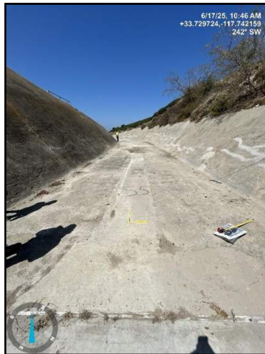
Photo 14) Spillway channel looking downstream. Note repairs of cracking on the right spillway wall and trench concrete in slab
