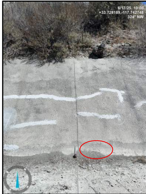
Photo 13) Previous concrete repairs throughout wall panels R8 and R9. 20”x 3”. Note concrete spall and debris.
