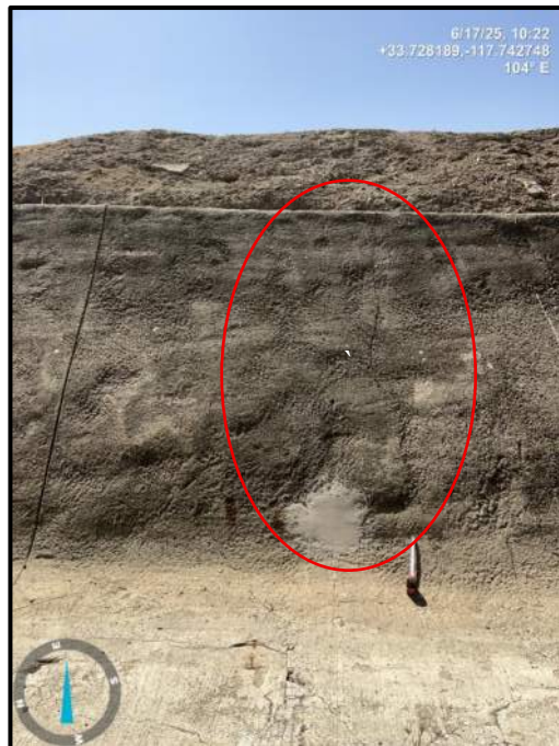
Photo 28) 1/4" longitudinal and transverse cracks on panel L16. Note recent concrete repair.
