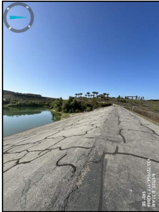
Photo 3) Dam crest, downstream face, and upstream face looking towards left abutment. Note minor cracking of AC liner.
