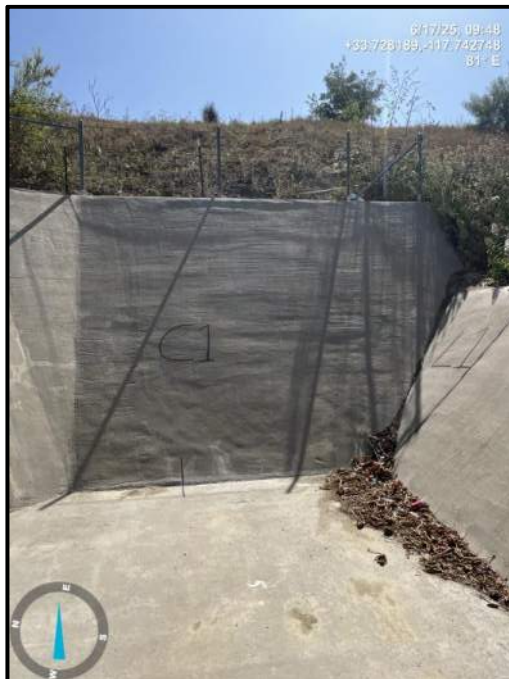
Photo 2) Wall panel C1 and L1. Note debris.
