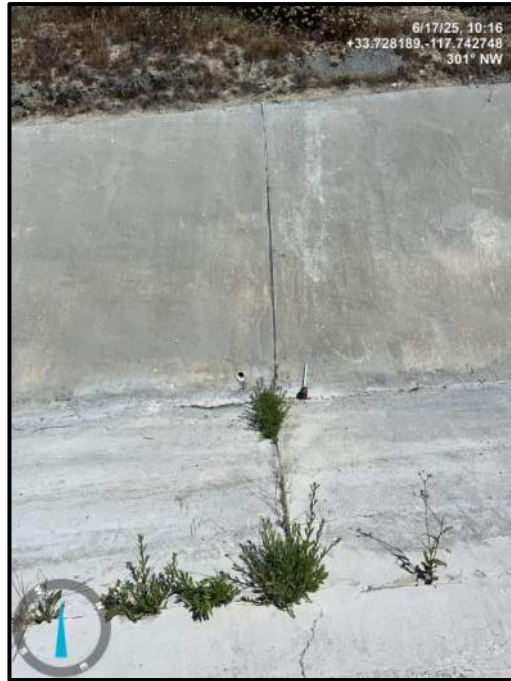
Photo 27) Vertical wall joint open 1/2" max between wall panels R15 and R16. Note slab joint open 1/2" max and vegetation in joint.
