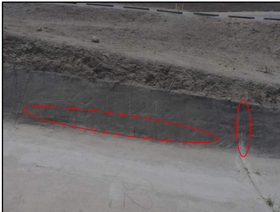
Photo 38) Bulge along wall panel L21. Note wall joint open ¼” max between wall panels L21 and L22.
