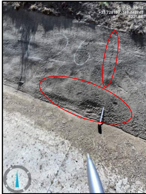
Photo 45) Concrete spall and ¼” longitudinal crack on wall panel L26. Note debris.
