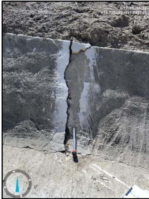
Photo 39) Crack open 1” max with 2” offset at wall panel L24.
