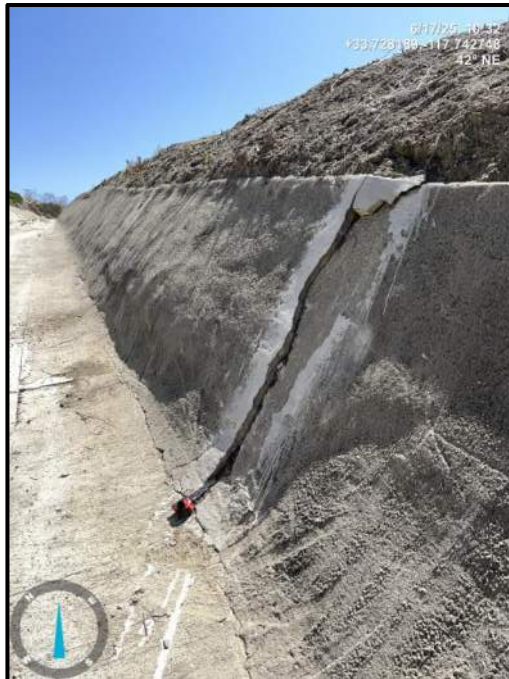
Photo 40) Crack open 1” max with 2” offset at wall panel L24.
