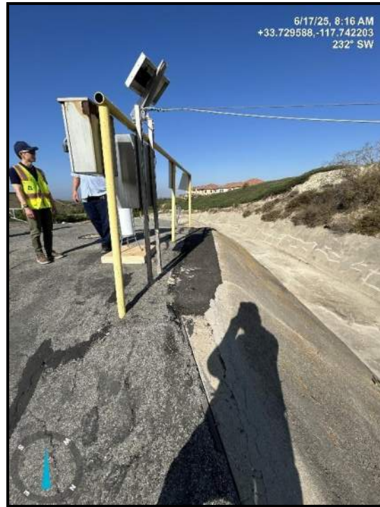
Photo 11) Recent repair of separation between AC pavement and spillway concrete liner joint.
