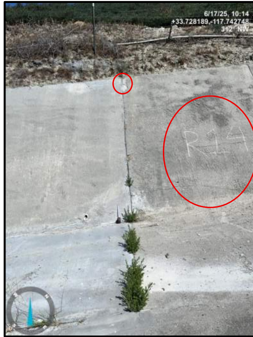
Photo 23) Vertical wall joint open \frac{1}{4} " max between wall panels R14 and R15 with 1" offset. Slab joint open \frac{1}{2} " max. Note concrete spall and cracks on wall panel R14, and vegetation growth along existing construction joint.
