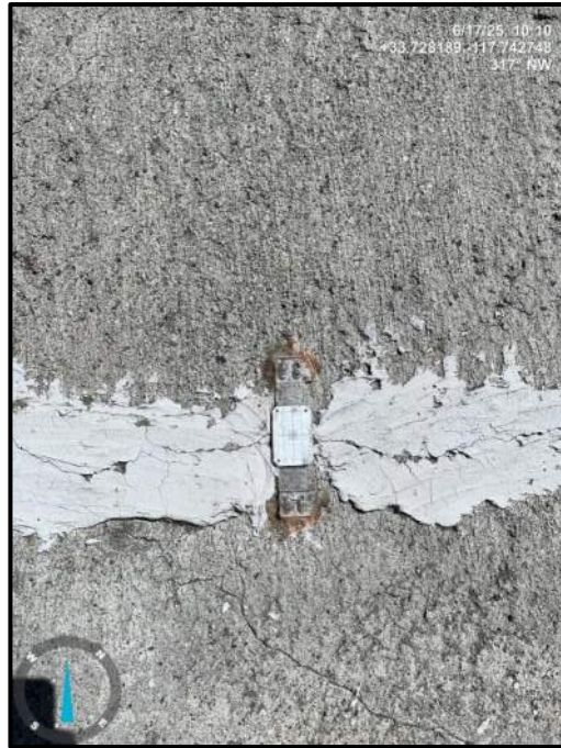
Photo 17) Existing crack gauge along crack at wall panel R11. Reading: North/South 1.00 mm and East/West -0.05 mm.
