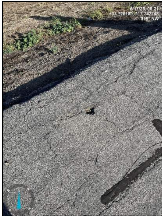
Photo 4) Minor cracking and popout in crest AC liner.
