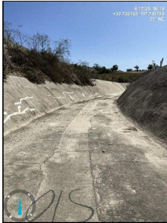
Photo 13) Spillway channel looking upstream. Note trench concrete and adjacent cracking.
