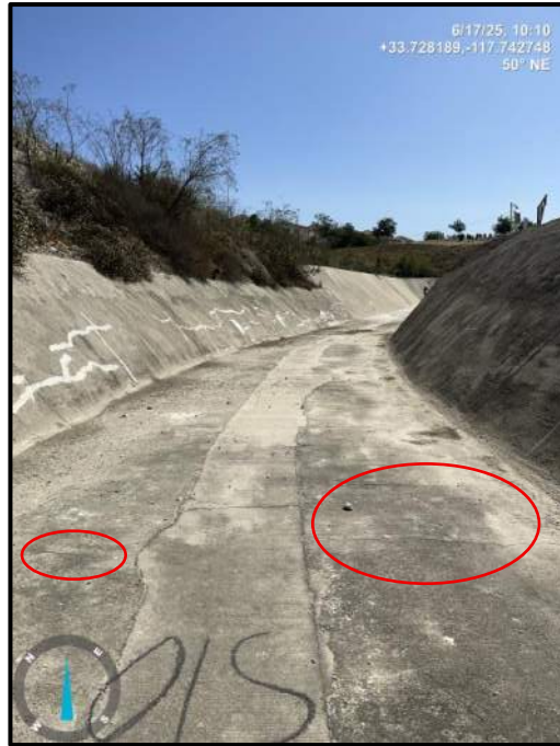
Photo 19) View of spillway and existing utility trench looking upstream. Note cracks along trench construction joints.
