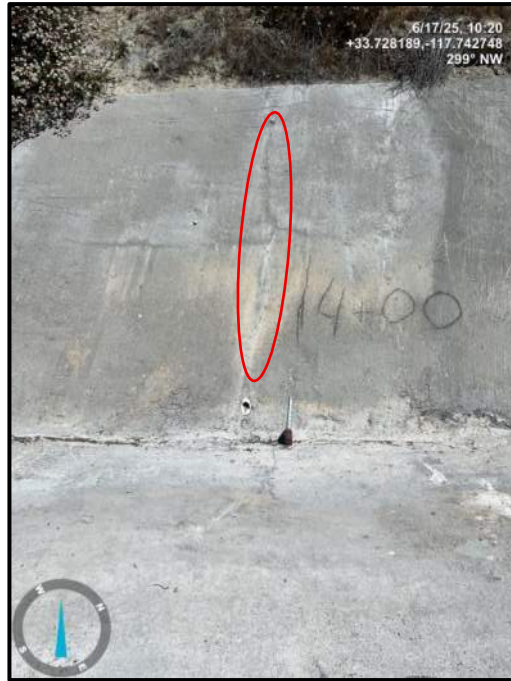
Photo 29) ¼” crack at panel R16. Note 2” diameter PVC weep hole.
