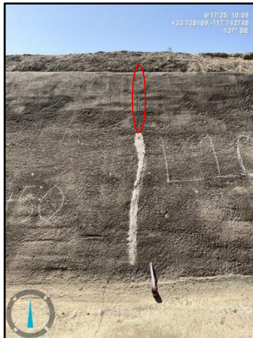
Photo 16) Delaminated previous repair and ¼” crack at wall panel L11.
