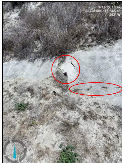
Photo 48) Vertical wall joint open \frac{1}{2} " max with 1 \frac{1}{2} " joint offset between wall panels R28 and R29. Note vegetation growth and \frac{1}{2} " transverse cracks.
