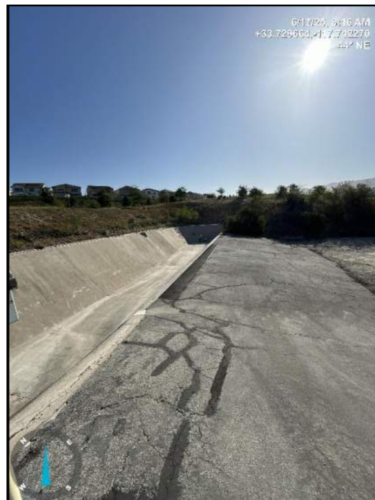
Photo 12) Spillway side channel looking upstream. Note recent repair at the AC line approach and spillway contact.
