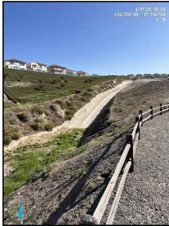
Photo 15) Spillway channel and stilling basin looking upstream. Note sediment and vegetation in stilling basin.
