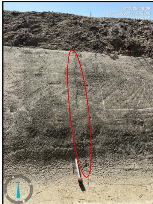
Photo 36) ¼" longitudinal crack on wall panel L20.
