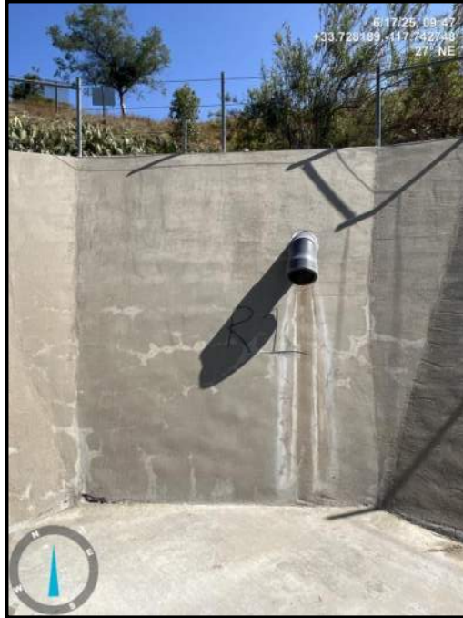
Photo 1) Wall panel R1. Note 10” PVC pipe and mineral precipitate.
