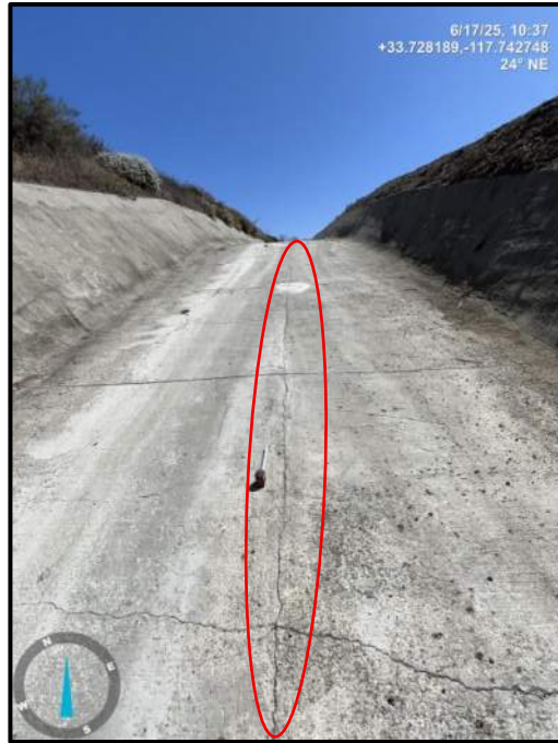
Photo 43) ¼” longitudinal and transverse cracks along spillway floor.
