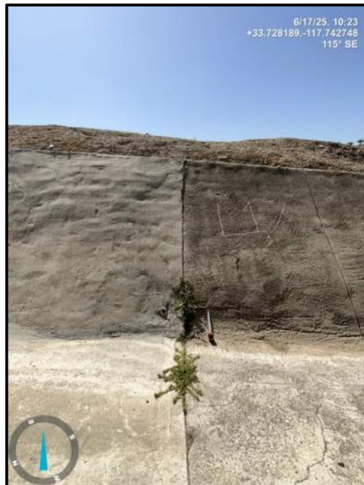
Photo 32) Vertical wall joint open 1" max with \frac{1}{2} " joint offset between wall panels L16 DS and L17. Note vegetation.
