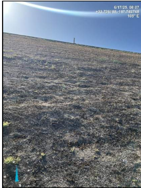
Photo 9) Rodent activity along right downstream face.
