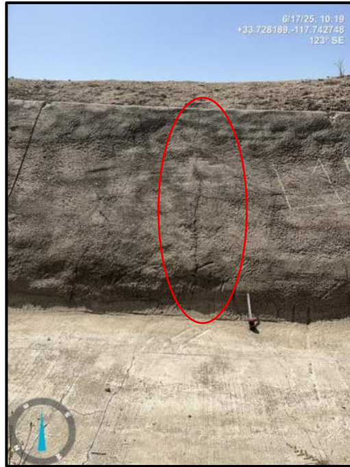
Photo 25) ½” longitudinal and transverse cracks along wall panel L15.
