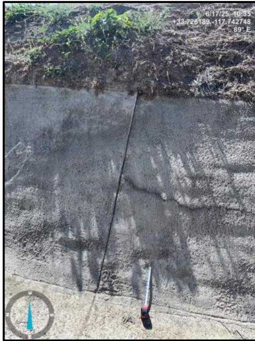
Photo 41) Vertical wall joint open \frac{1}{2} " max with \frac{1}{4} " joint offset between wall panels L25 and L26. Note \frac{1}{2} " transverse crack.
