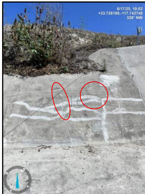
Photo 10) Previous repairs throughout panel R6. Note 1/4" cracks and vegetation covering top of panel.
