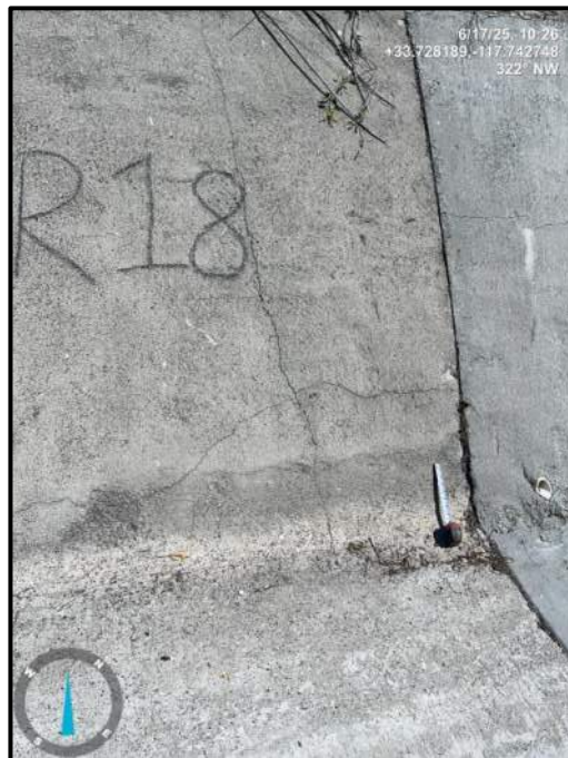
Photo 34) Vertical wall joint open ½” max with 1” joint offset between wall panels R17 and R18. Note longitudinal and transverse cracks.
