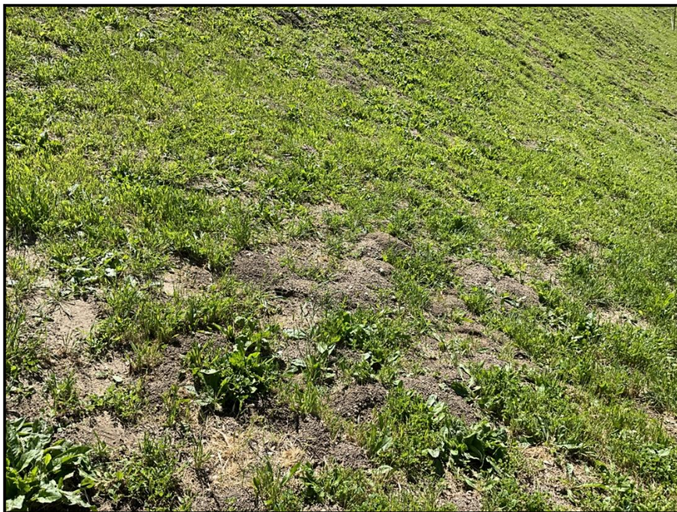
Photo 7) Rodent activity along left downstream face.
