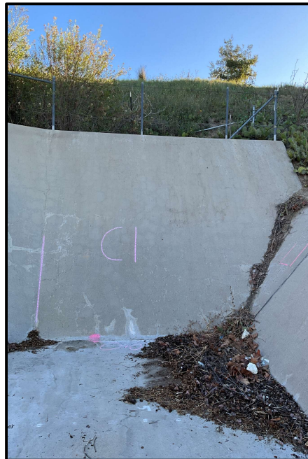
Photo 2) Wall panel C1 and L1. Note debris.
