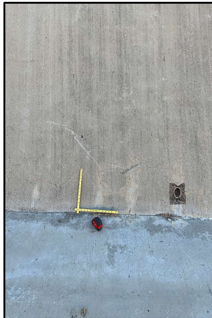
Photo 4) Typical 3”diameter weep hole. Note concrete popout.
