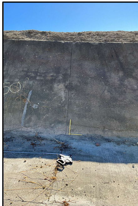
Photo 26) Wall joint open \frac{1}{2} " max between wall panels L14 and L15. Note \frac{1}{2} " longitudinal crack, concrete spalling, and delaminated previous repair.
