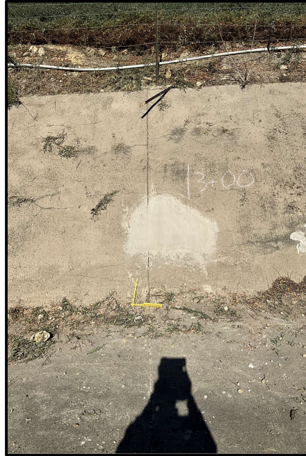
Photo 21) Wall joint open \frac{1}{4} " max between wall panels R12 and R13. Note previous concrete repair
