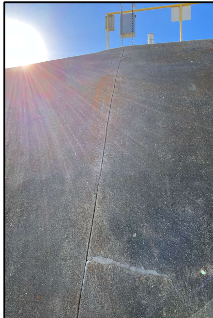
Photo 12) Wall joint open 1/4" max between wall panels L6 and L7. Note delaminated previous concrete repair and 1/4" cracks.
