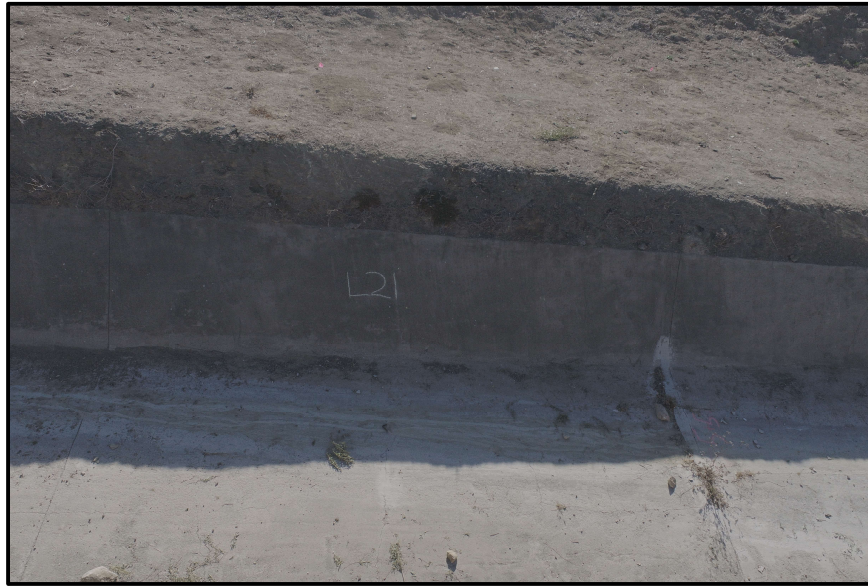
Photo 35) Bulge along wall panel L21. Note wall joint open \frac{1}{4} " max between wall panels L21 and L22.
