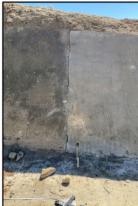
Photo 30) 1" D/S projecting wall joint open \frac{1}{4} " max between wall panels L16 US and L16 DS. Note \frac{1}{2} " longitudinal cracks and concrete popout.
