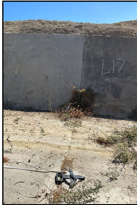
Photo 31) ½" U/S projecting wall joint open 1" max between wall panels L16 DS and L17. Note vegetation growing in wall and slab joints.
