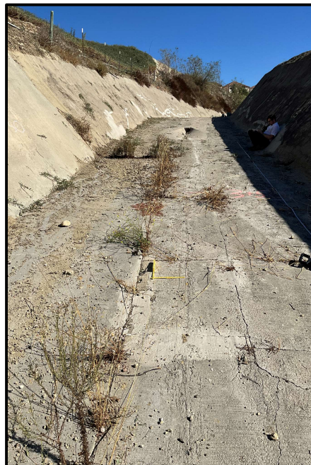
Photo 24) Existing trench from previous spillway channel repairs looking U/S. Note cracks and vegetation along construction joints.
