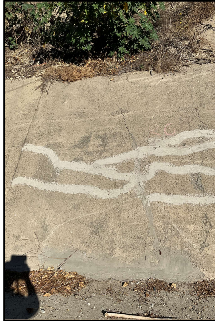
Photo 11) Panel R6. Note delaminated concrete repairs and 1/4" cracks. Note debris.
