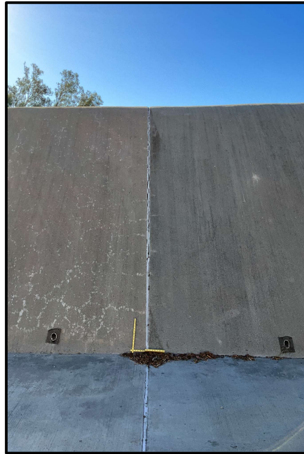
Photo 7) Wall joint open 1/2" max between wall panels L4 and L5.
