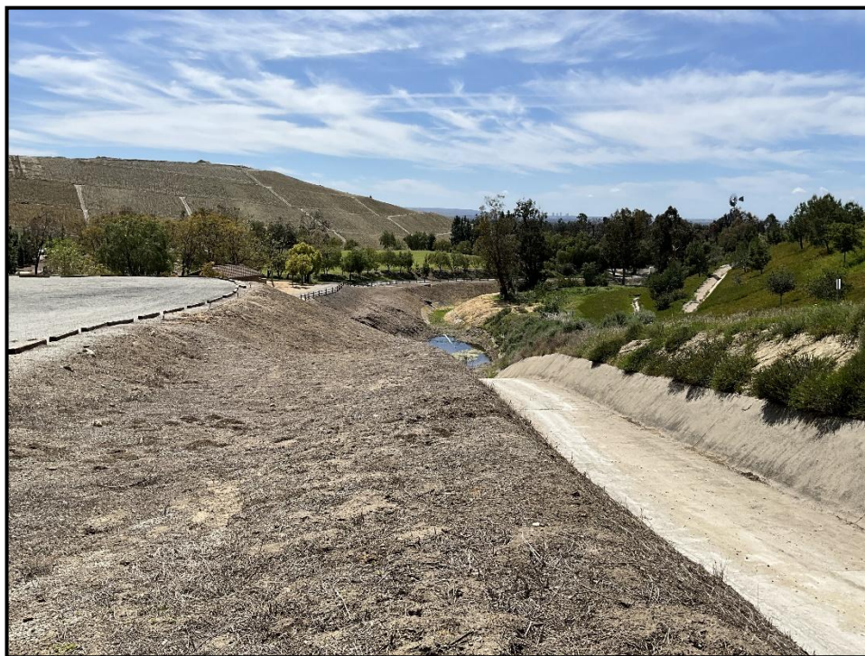
Photo 11) Spillway channel. Note hairline cracking on the right spillway wall.
