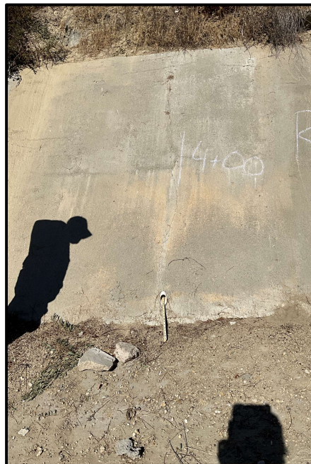
Photo 28) \frac{1}{4} " crack at panel R16. Note 2" diameter PVC weep hole.
