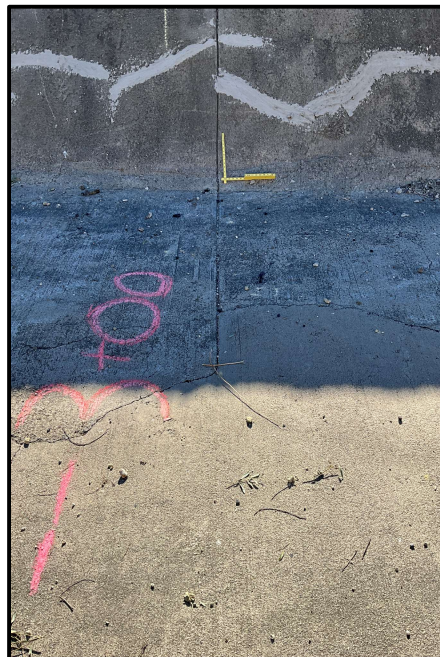
Photo 20) ¼" max slab joint opening and wall joint opening at wall panels L13 and L14. Note utility trench construction joints.
