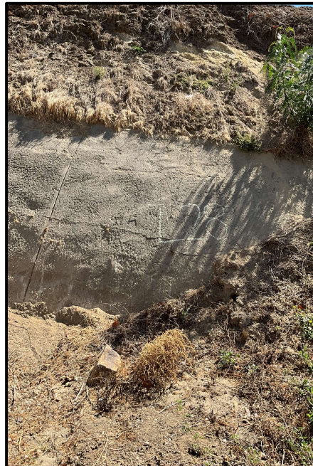
Photo 44) ½" transverse crack along wall panel L28.
