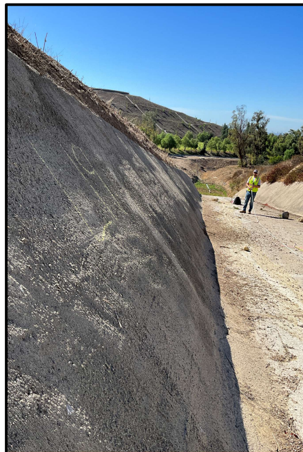
Photo 32) Bulge along wall panels L19, L20, and L21.
