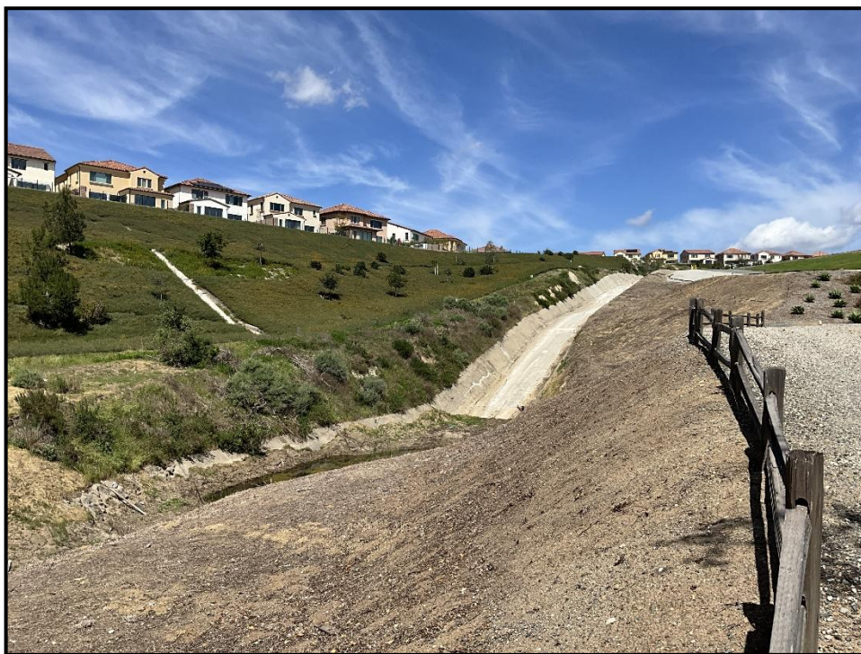
Photo 12) Hairline cracking on right spillway wall. Note crack gauge on longitudinal crack.
