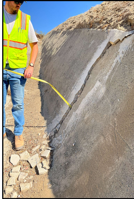
Photo 37) 2" U/S projecting wall crack open 1" max at wall panel L23.
