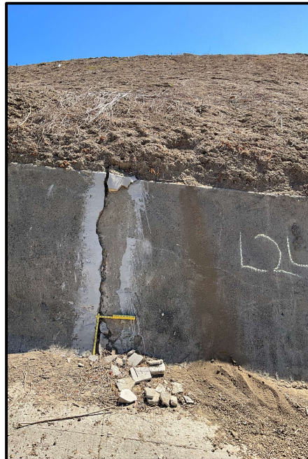
Photo 38) 2" U/S projecting wall crack open 1" max at wall panel L24.
