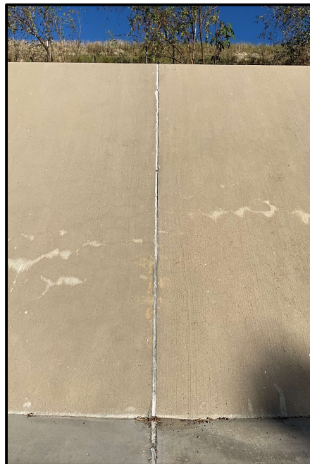
Photo 8) Wall joint open 1/2" max between wall panels R4 and R5. Note recent concrete repairs.
