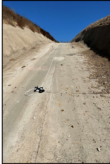
Photo 41) ½” longitudinal crack along spillway floor.
