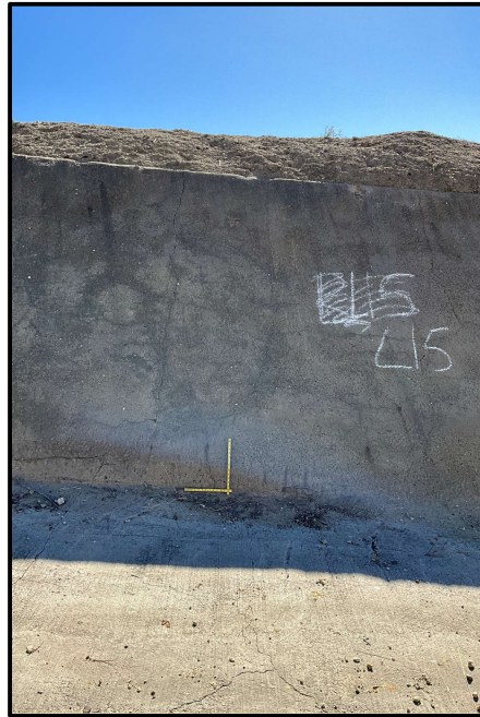
Photo 27) \frac{1}{2} " longitudinal and transverse cracks along wall panel L15. Note concrete spalling at bottom of wall.
