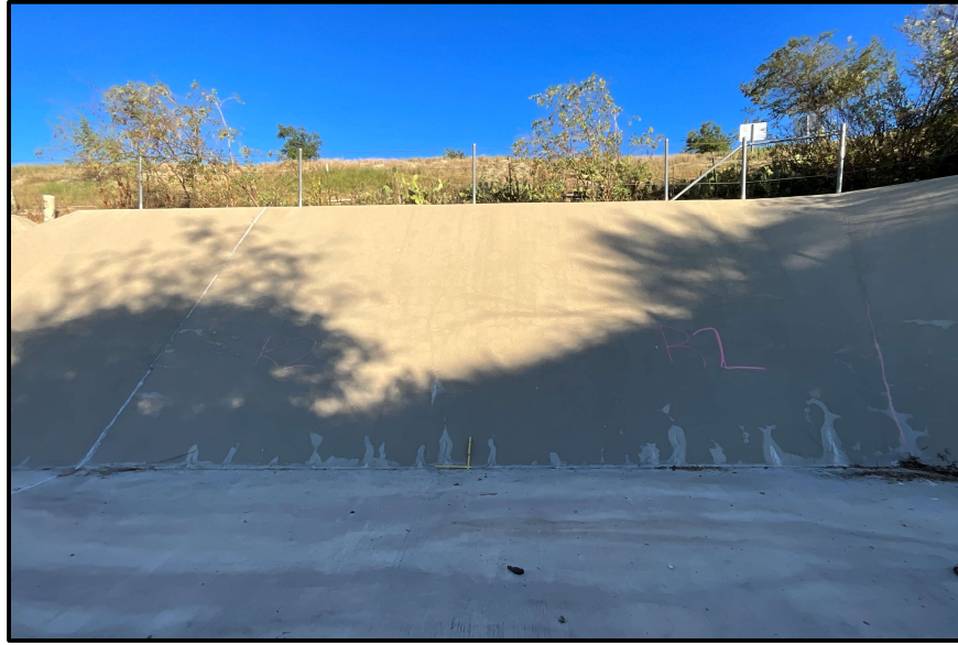
Photo 5) Wall panel R2. Wall joint open \frac{1}{2} " max between wall panel R2 and R3. Note previous concrete repairs.
