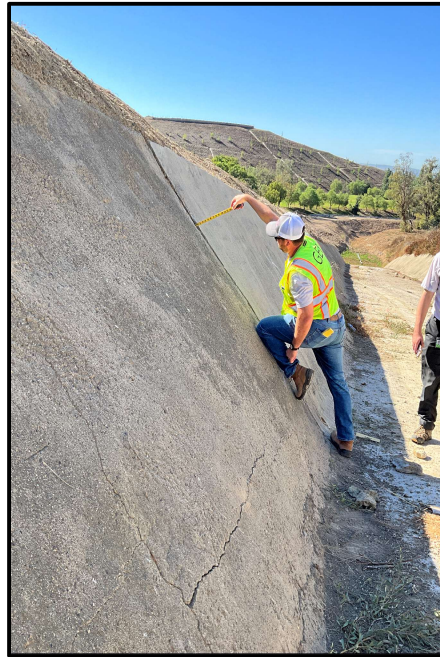
Photo 29) 1" D/S projecting wall joint open \frac{1}{4} " max between wall panels L16 US and L16 DS. Note \frac{1}{2} " longitudinal cracks.
