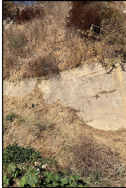
Photo 43) 1 ½" D/S projecting wall joint open ½" max between wall panels R28 and R29. Note vegetation growing in wall joint and ½" transverse cracks.
