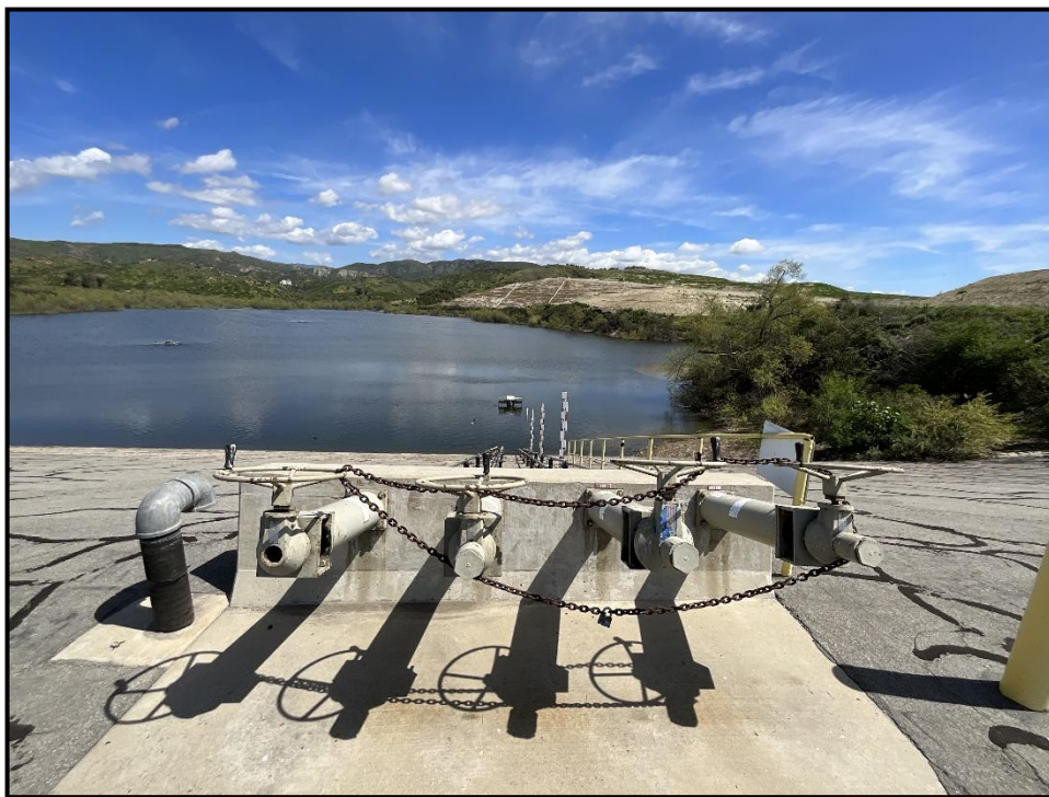
Photo 14) Upstream outlet valves.
