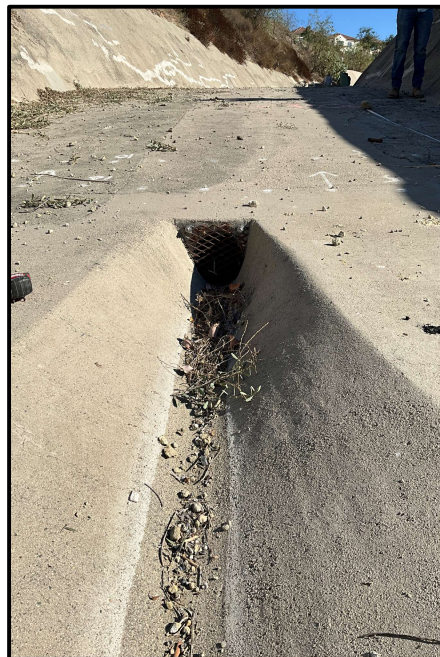
Photo 22) 8" diameter PVC spillway drain looking U/S. Note debris.
