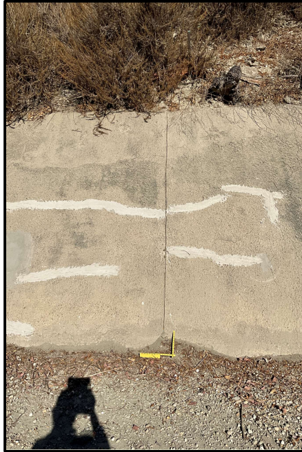
Photo 13) Previous concrete repairs (typ) wall panels R8 and R9. Note debris.
