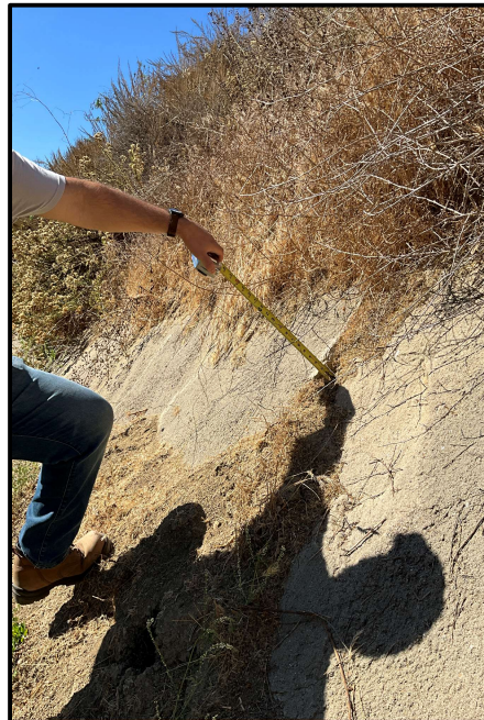
Photo 42) 1 ½” D/S projecting wall joint open ½” max between wall panels R28 and R29. Note vegetation growing in wall joint.
