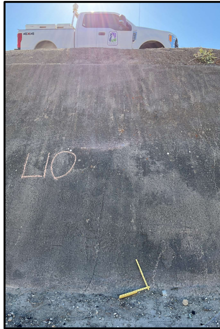
Photo 15) ¼" crack at wall panel L10.
