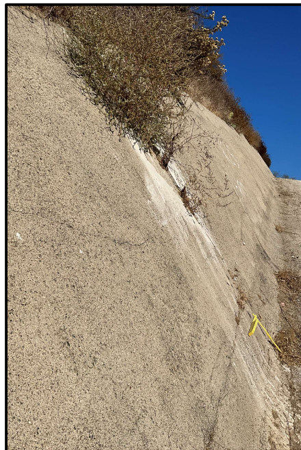
Photo 40) 1 ¾" U/S projecting wall joint open ½" max between wall panels R25 and R26. Note vegetation growing in wall joint
