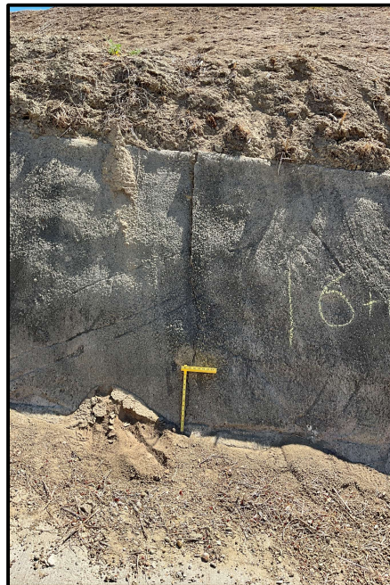
Photo 36) \frac{1}{2} " D/S projecting wall crack open \frac{1}{4} " max at wall panel L23.
