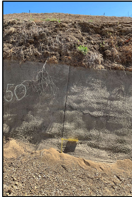
Photo 39) ¼" U/S projecting wall joint open ½" max between wall panels L25 and L26. Note ½" transverse crack.
