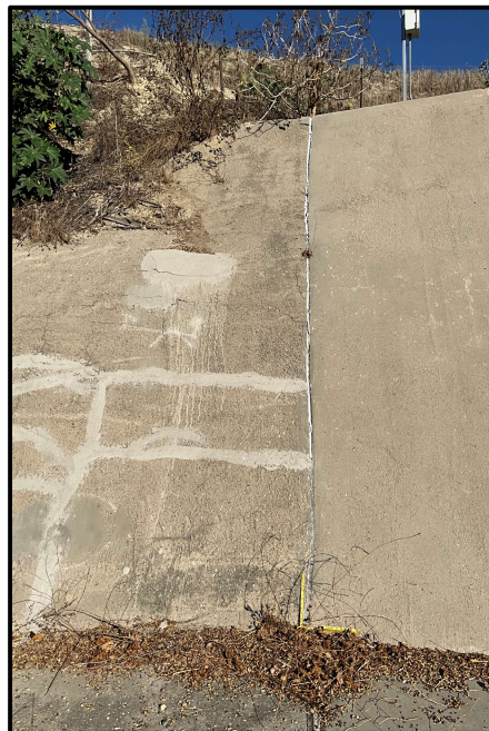
Photo 10) Wall joint open 1/2" top to middle between wall panels R5 and R6. Note delaminated previous concrete repair and 1/4" cracks. Note debris.
