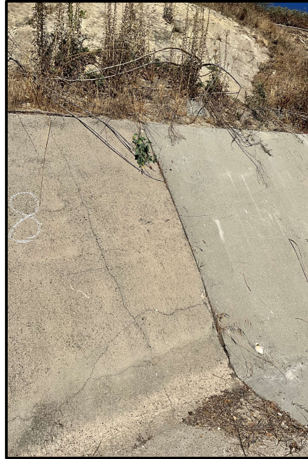
Photo 33) 1" U/S projecting wall joint open \frac{1}{2} " max between wall panels R17 and R18. Note vegetation growing in wall and slab joints.
