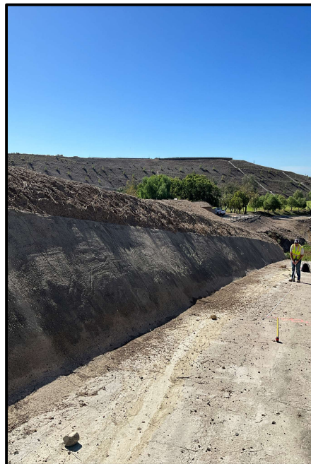
Photo 34) Bulge along wall panels L19, L20, and L21. Note \frac{1}{4} " transverse crack.
