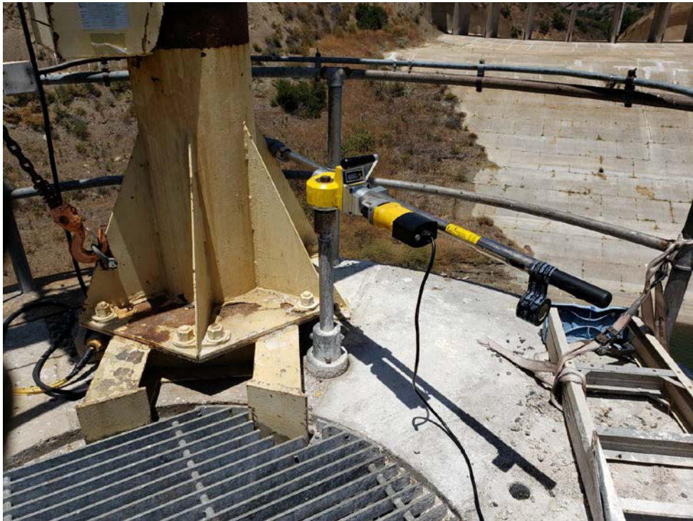
The four upstream valves in the outlet tower were fully cycled.
