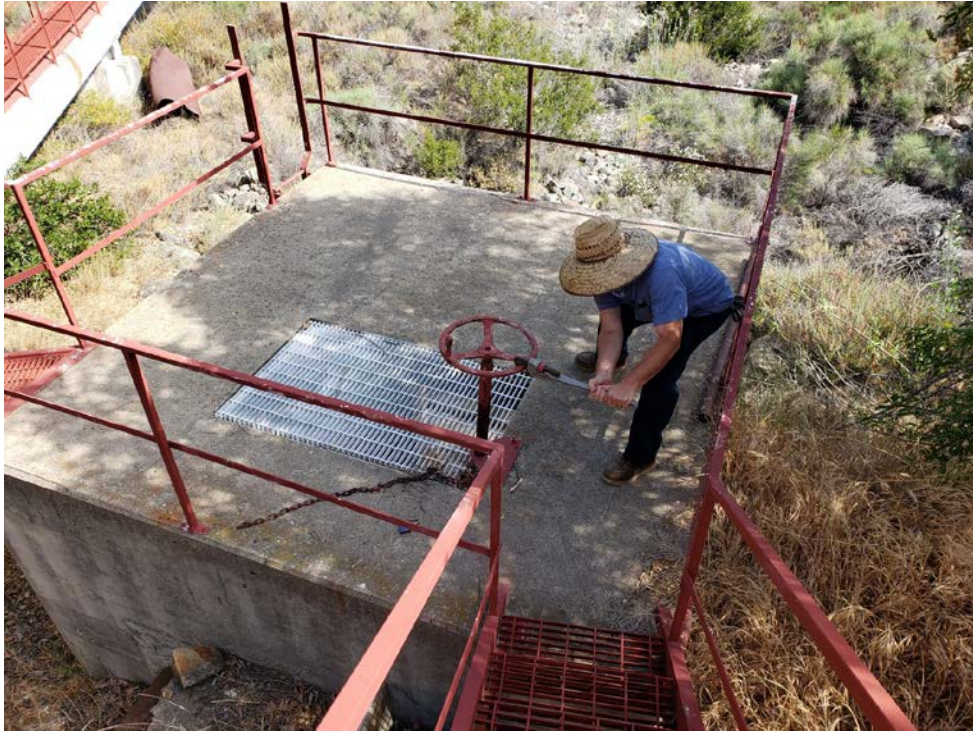
The downstream blowoff valve was fully cycled.
