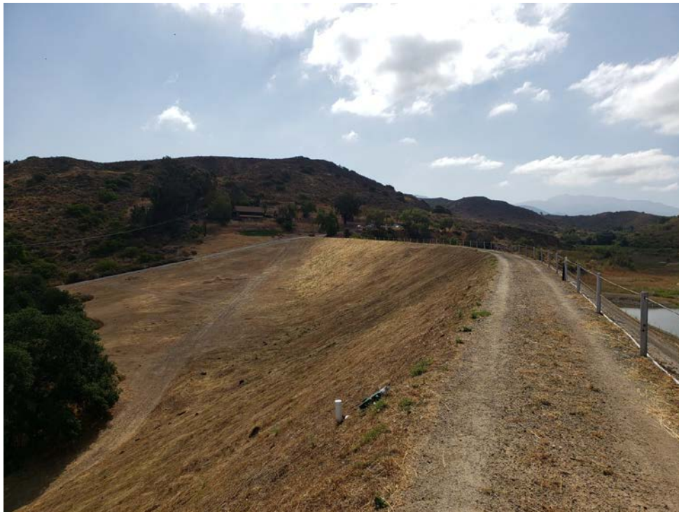
View of the crest and downstream slope looking towards the right abutment.
