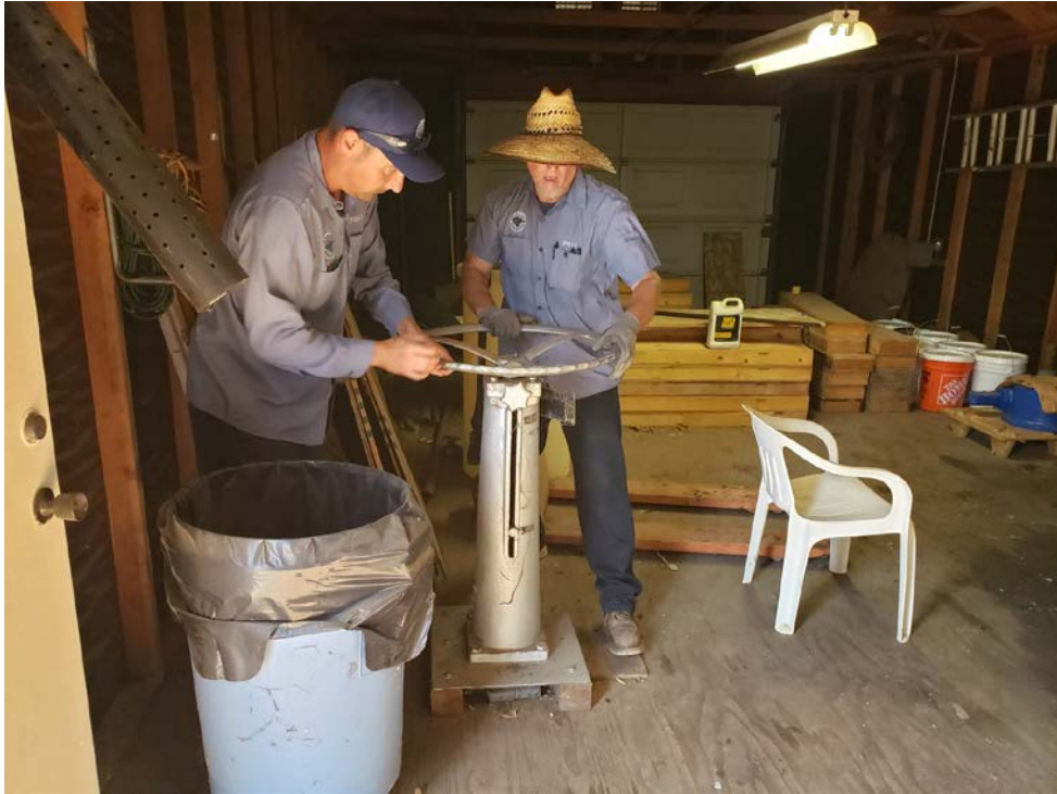
The downstream diverter valve in the outlet house was fully cycled.
