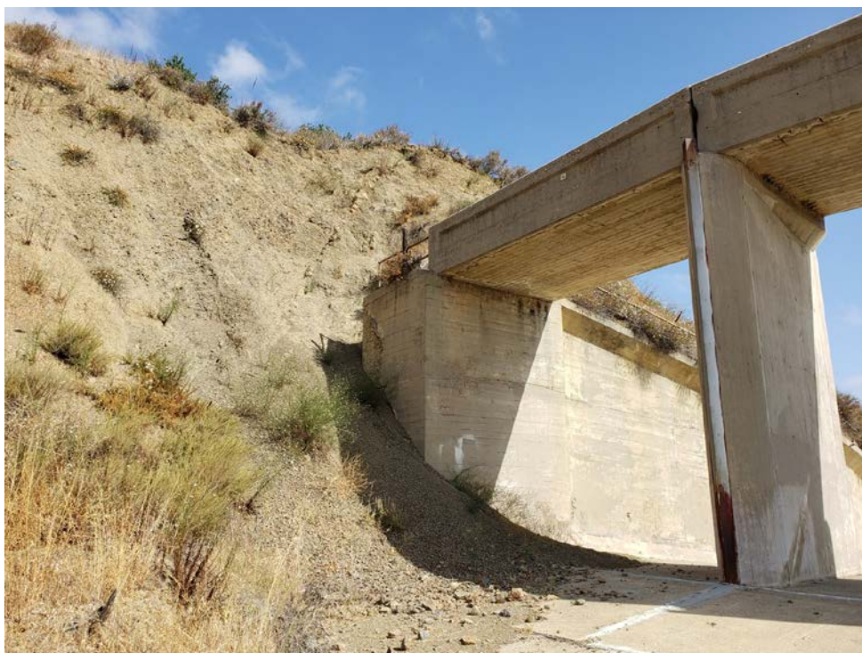
The interface between the upper left abutment and spillway continues to erode.
