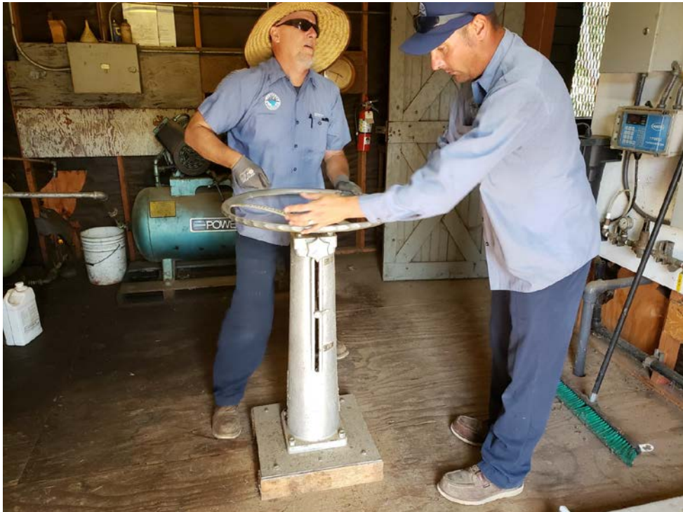
The main service valve was cycled 50% due to water demands.
