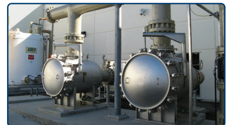
Filters to prevent sand or silt from entering reverse osmosis trains.
