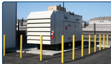
Diesel-powered emergency generator.
