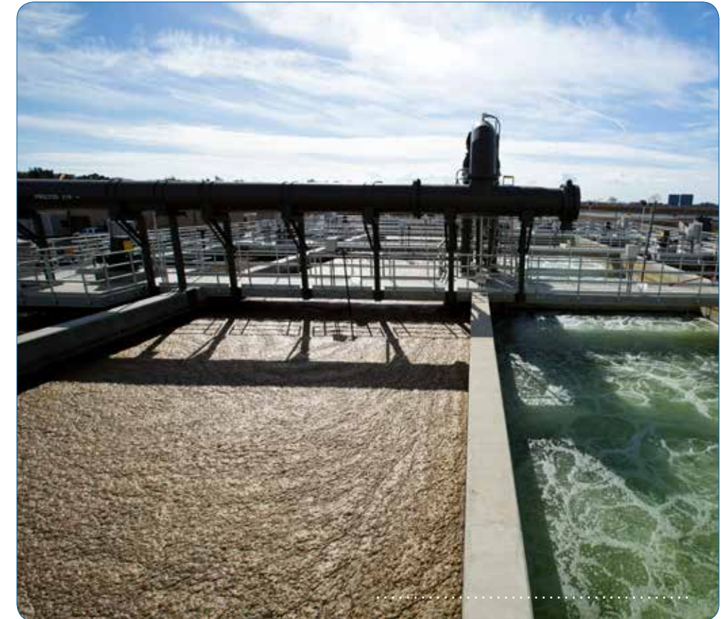
Treatment basins for the cutting-edge membrane bio-reactor process at Michelson Water Recycling Plant, part of the recent Phase 2 expansion of this facility.
