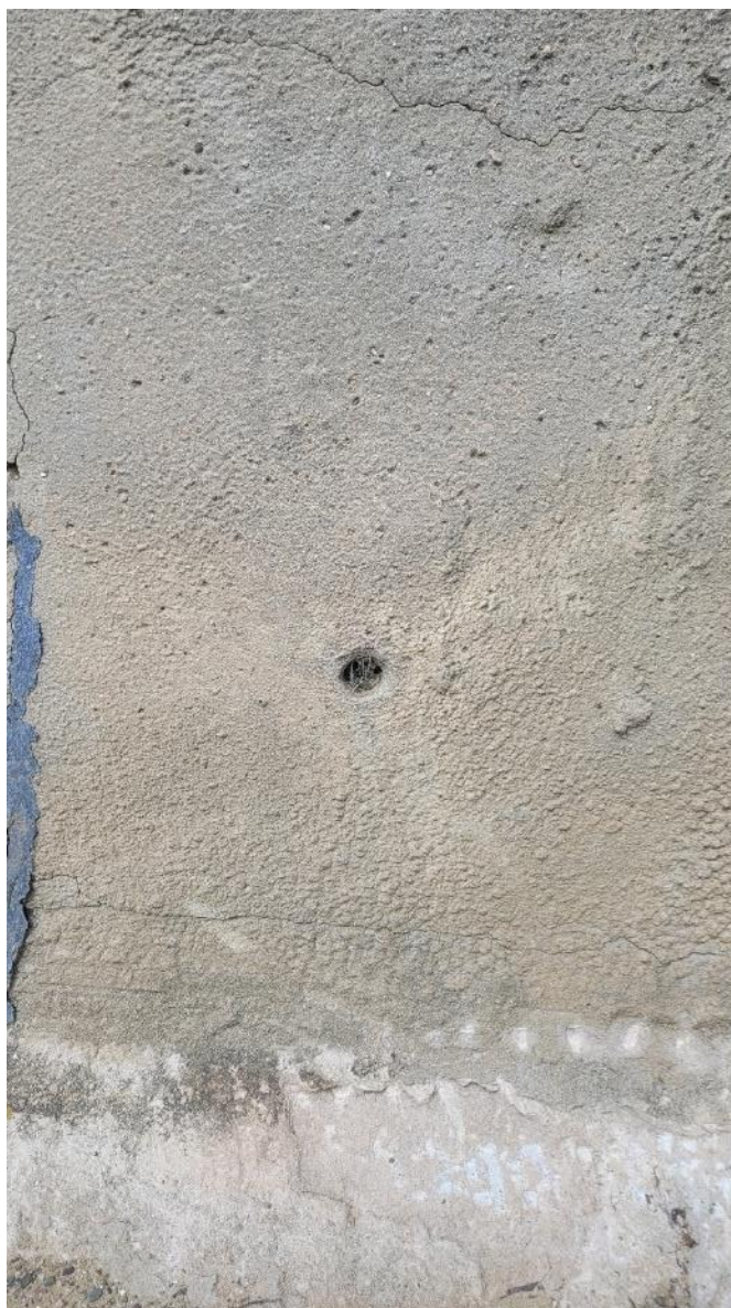
Photo 1: View of debris in one of the spillway weepholes.
