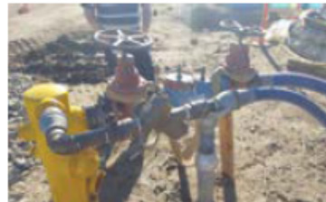
Another meter with backflow assembly
