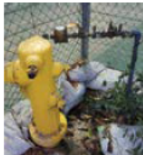
Meter with backflow assembly
