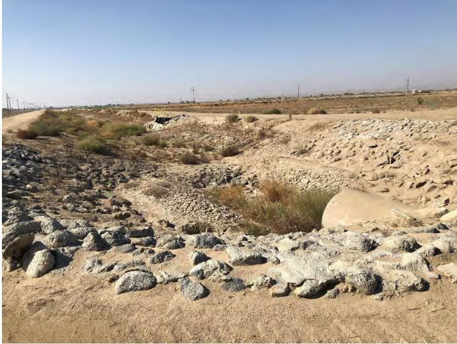
Photo 3: View looking south at the CVC outlet to the South Strand feeder canal. Silt buildup can be seen on either side of the outlet pipe.
