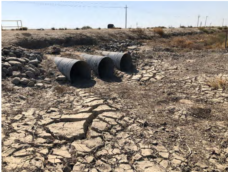
Photo 4: View of South Strand Basin 4 inlet pipelines showing buildup of silt near the pipes.
