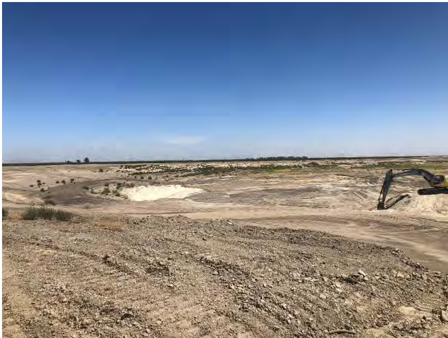
Photo 7: Deepening of basins at the Buena Vista Water Storage District Daly Ranch Facility.
