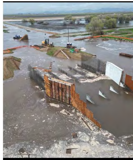
Friant-Kern Canal Breach, March 11, 2023
