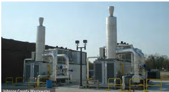
Johnson County Wastewater
