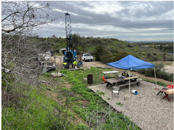
Tri-County Drilling and AECOM have worked together on many dam projects in Southern California – Syphon Reservoir
