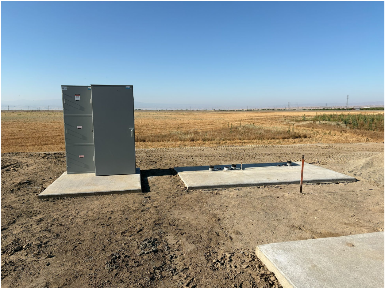
Meter Panel Installed at SN-1
