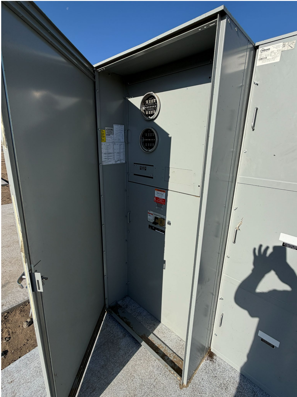
Meter Panel Installed at WE-1
