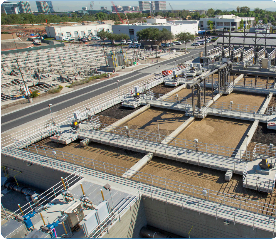
Treatment basins for the cutting-edge membrane bioreactor process at Michelson Water Recycling Plant, part of the recent expansion of this facility.
