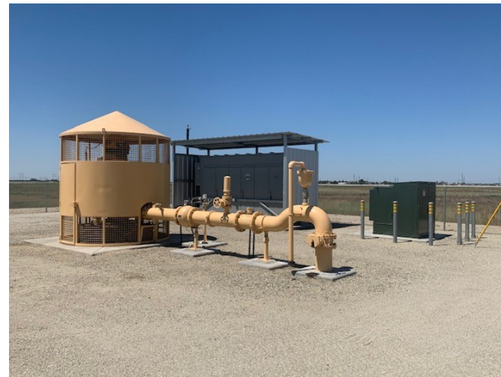
Typical Well Site
