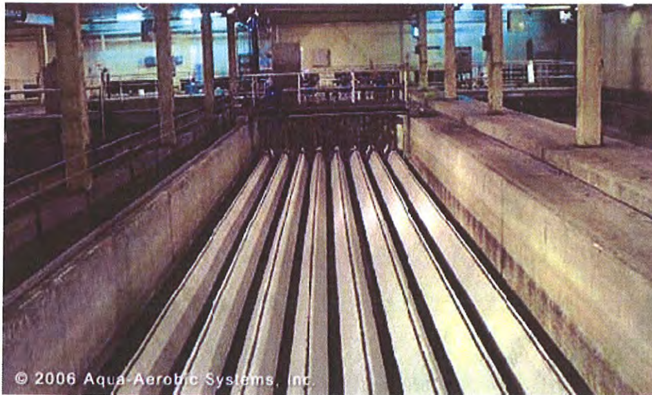
Figure 5-6: AquaDiamond Cloth Filter Installation
