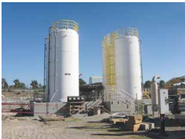
The Phase 2 Expansion of IRWD's Michelson Water Recycling Plant reached its first major milestone with the completion of a new disinfection facility featuring these two large sodium hypochlorite containers.
