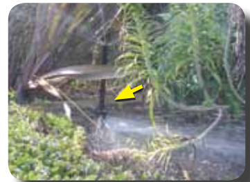
To prevent over-watering watch for leaks like this.
