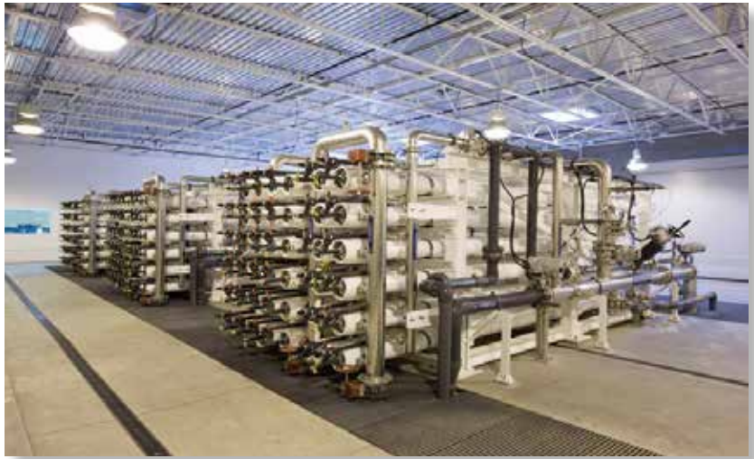
Wells 21 & 22 Water Treatment Plant
