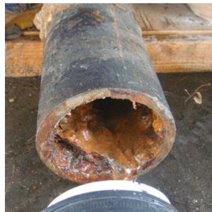
Figure 4-4. Tuburculated CI Pipe in testing for CalAM Monterey
