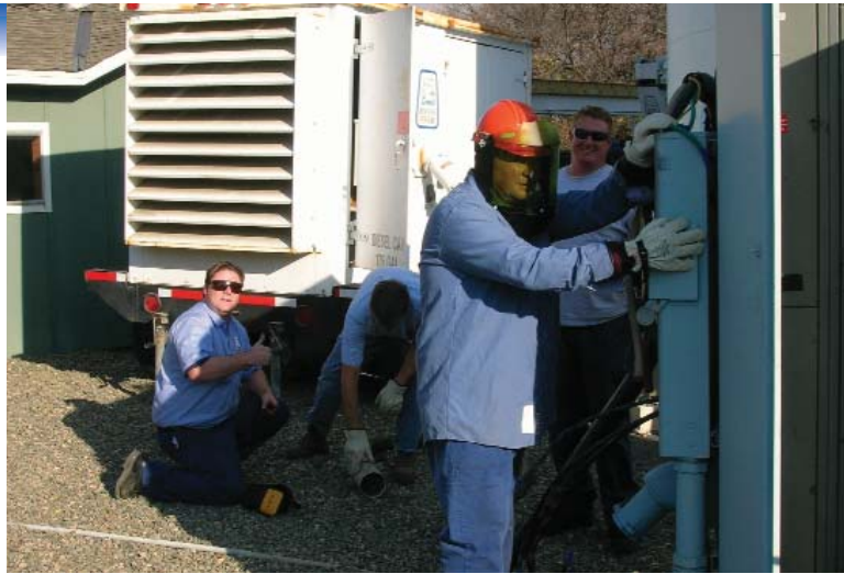
IRWD crews set up generators to keep water pumps operating after fire knocked out power in Silverado Canyon.
