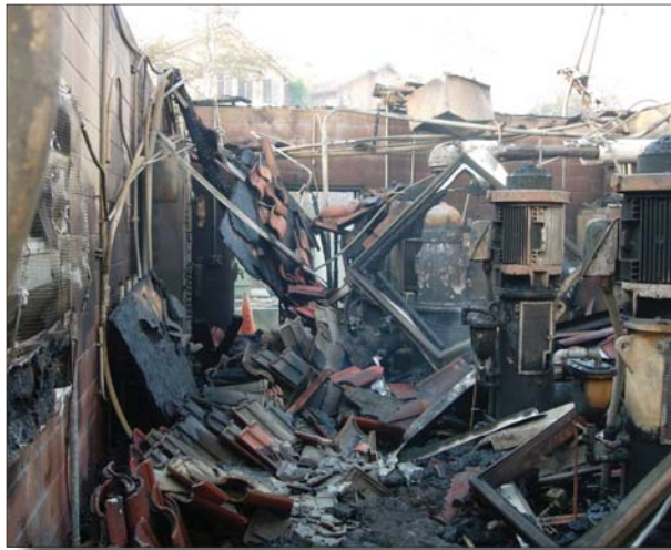
The Portola Hills Zone 9 Pump Station was reduced to a pile of rubble during the Santiago Fire.
